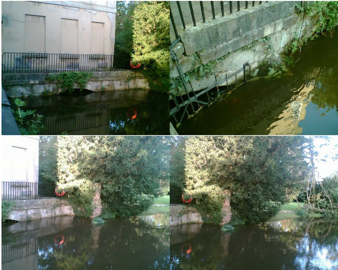
Figure 10: Photos of the flooding at Grandpont House in 2007.
