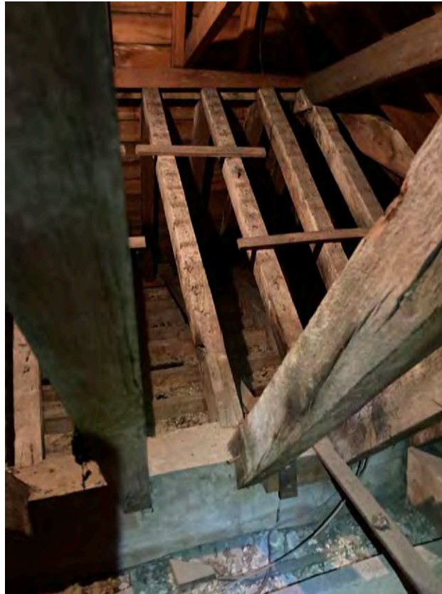
3.38 The interior of the roof to the west wing showing the retained 18C structure
