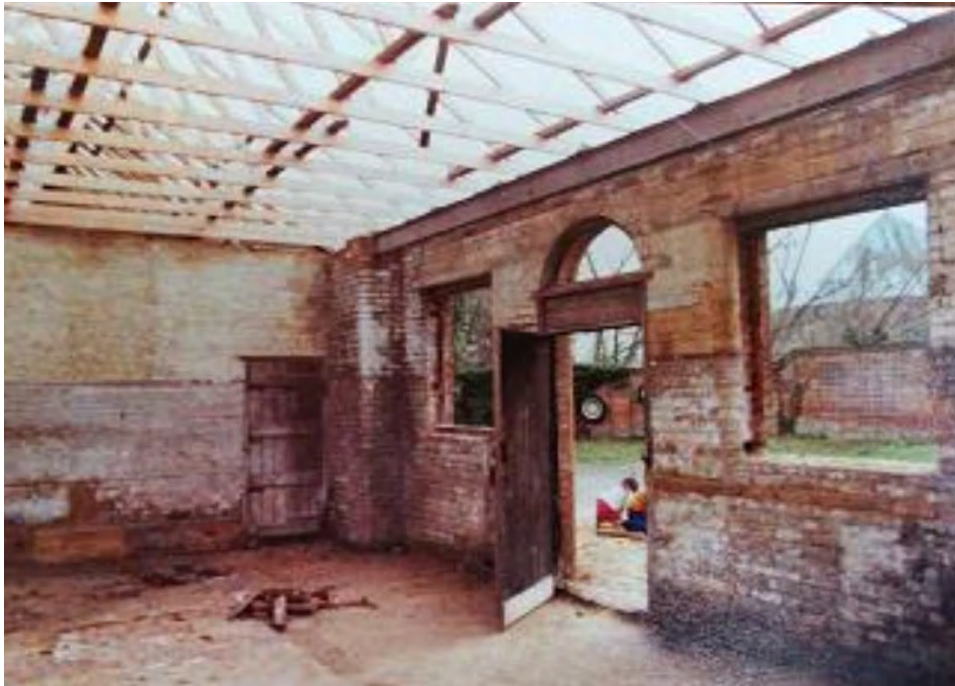
2.23 Replacement of the stable block roof from the central bay, c.1976 (Grandpont House archives)
