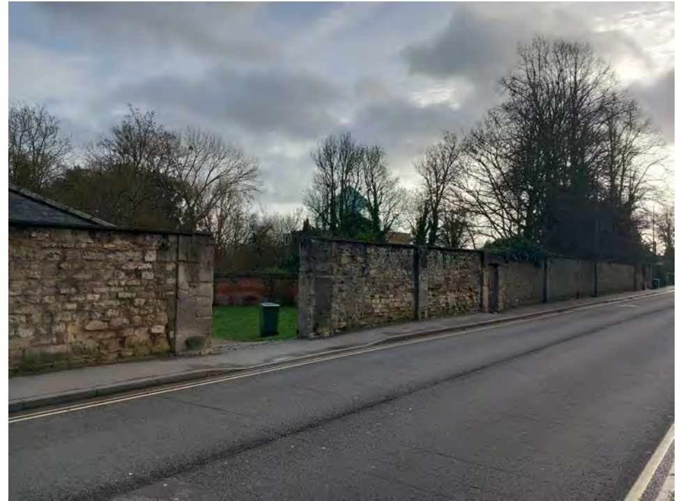
3.50 The garden wall on Abingdon Road. The entrance to the courtyard is on the left, and the pedestrian entrance on the right.
