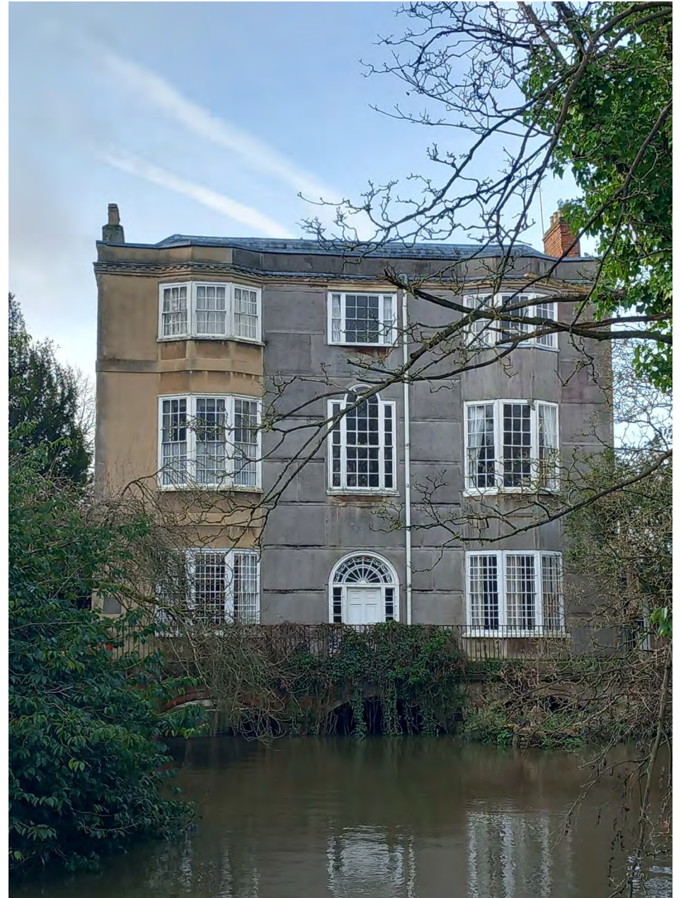
2.6 The east front of the east wing, showing the arches on which the house is built across the Isis (DIA)
