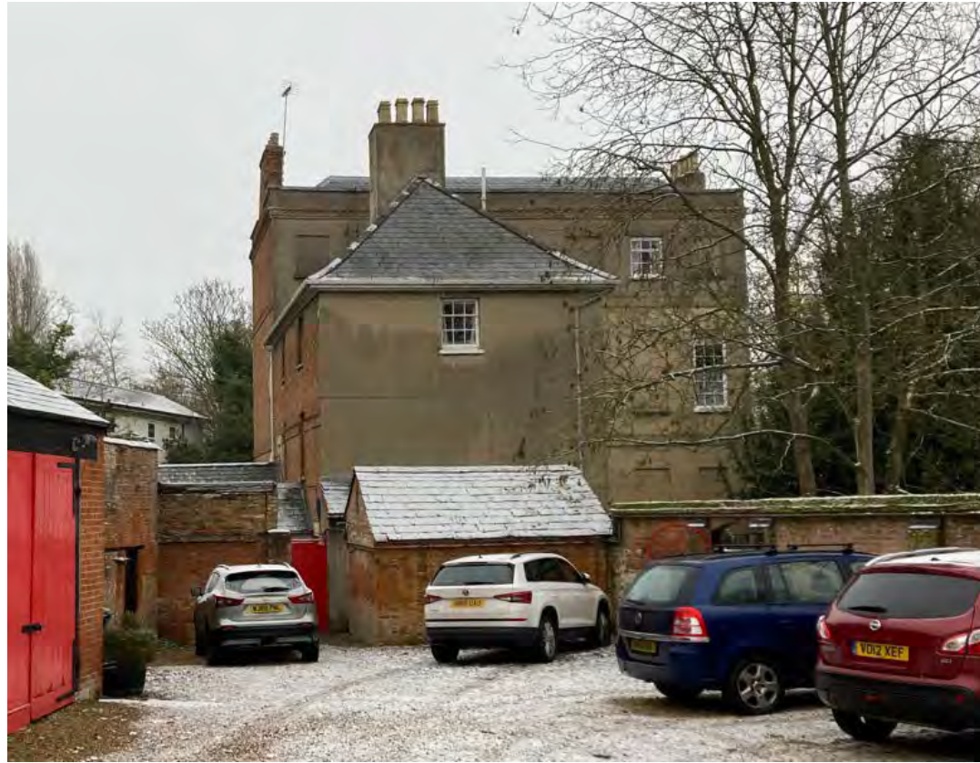
3.10 The west wall of the west wing, seen from the entrance courtyard, with the main house behind
