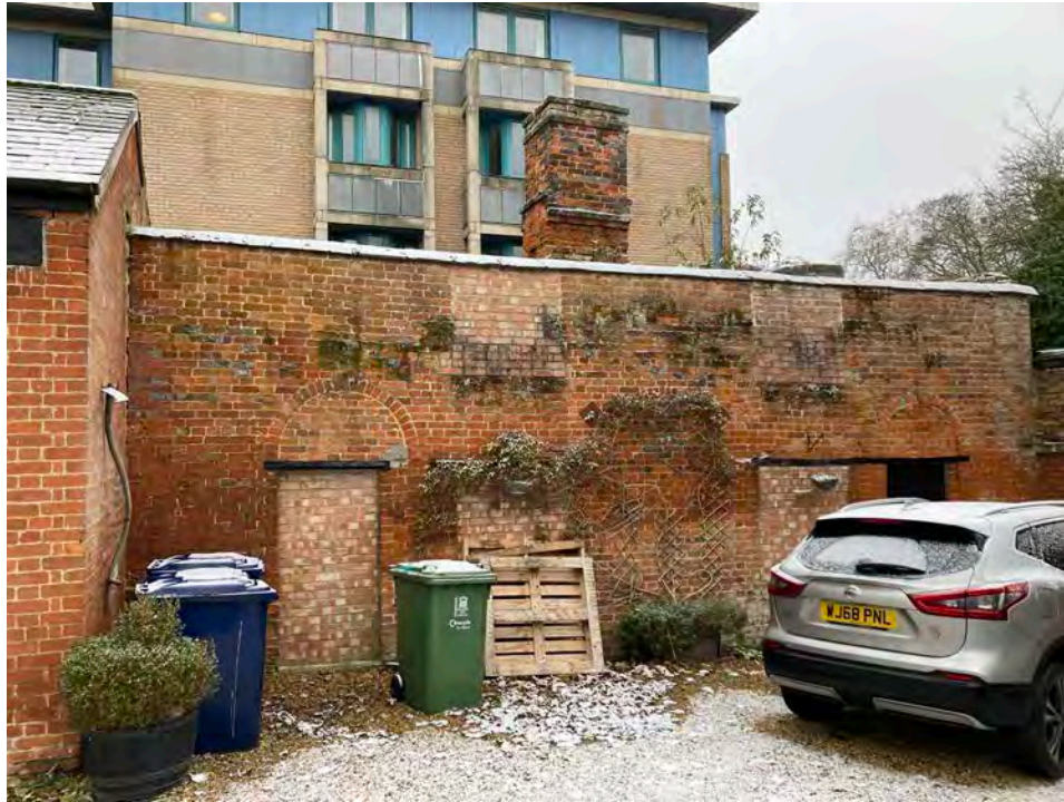
3.17 The south facade of the derelict cottages
