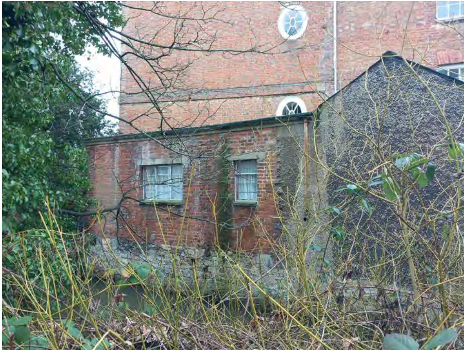
3.13 The north wall of the extensions on the north side of the main house
