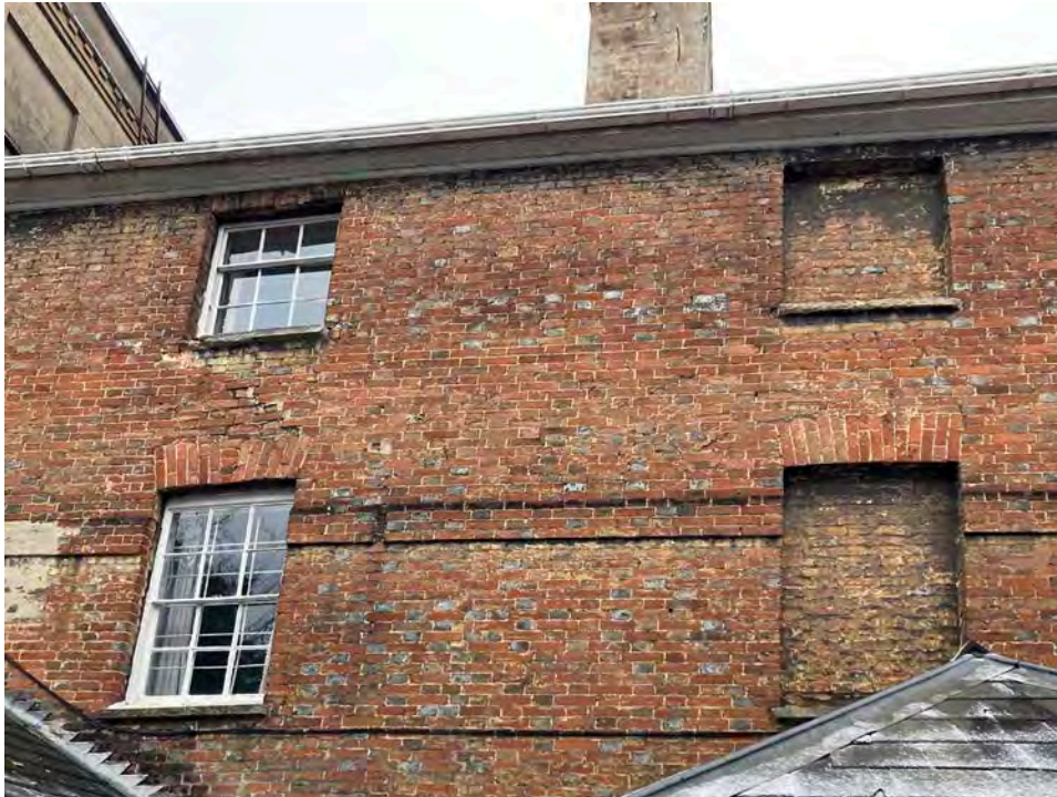
3.11 The north wall of the west wing
