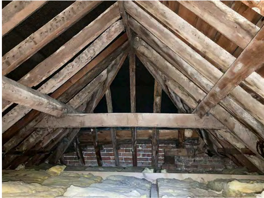
3.8 The interior of the western roof of the east wing looking east
