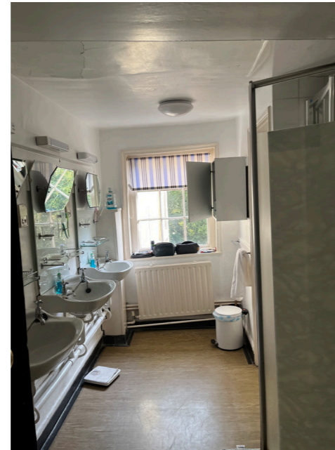
Image 16: Internal view of west wing 20th c. communal bathroom at first floor
