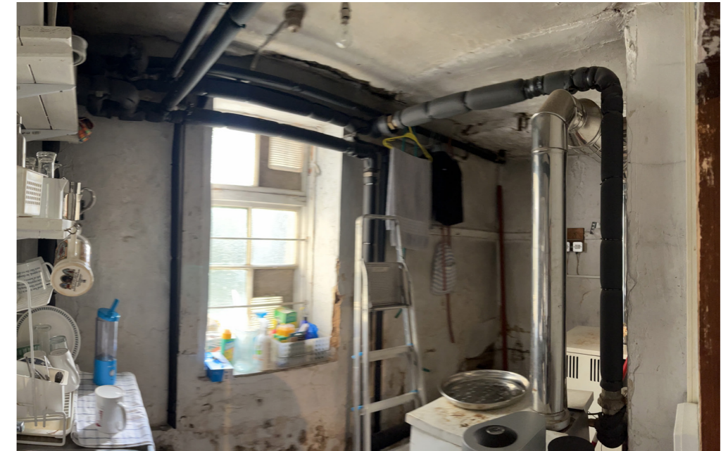
Image 18: Internal view of west wing 20th c. Boiler room addition at ground floor
