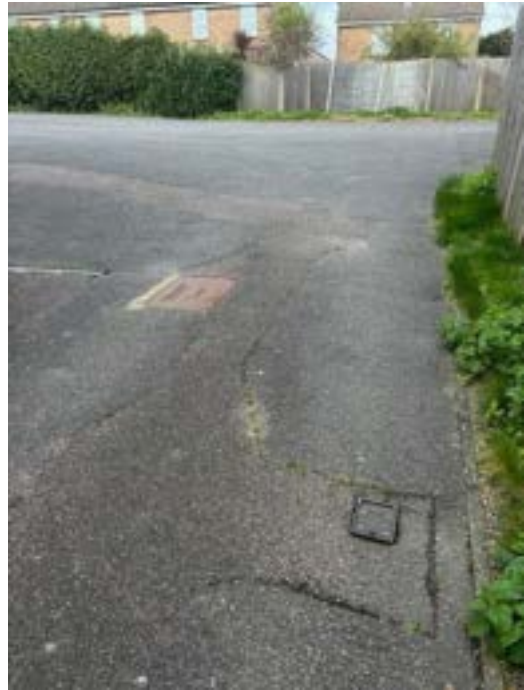
Photo 10: View from access road to car park-typical repair work round service inspection covers
