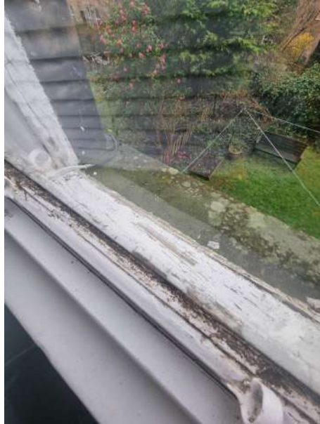
Photo shows the seals to the glass have failed which is allowing water to enter the woodwork and making the windows not efficient. The photo also shows the rotting sill externally.
