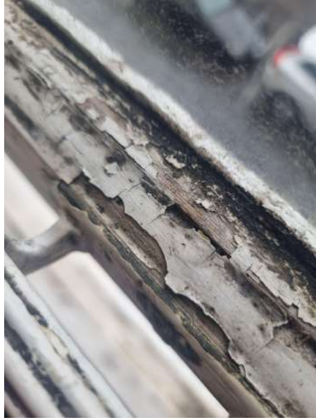
Deteriorated woodwork to the bottom rail.
