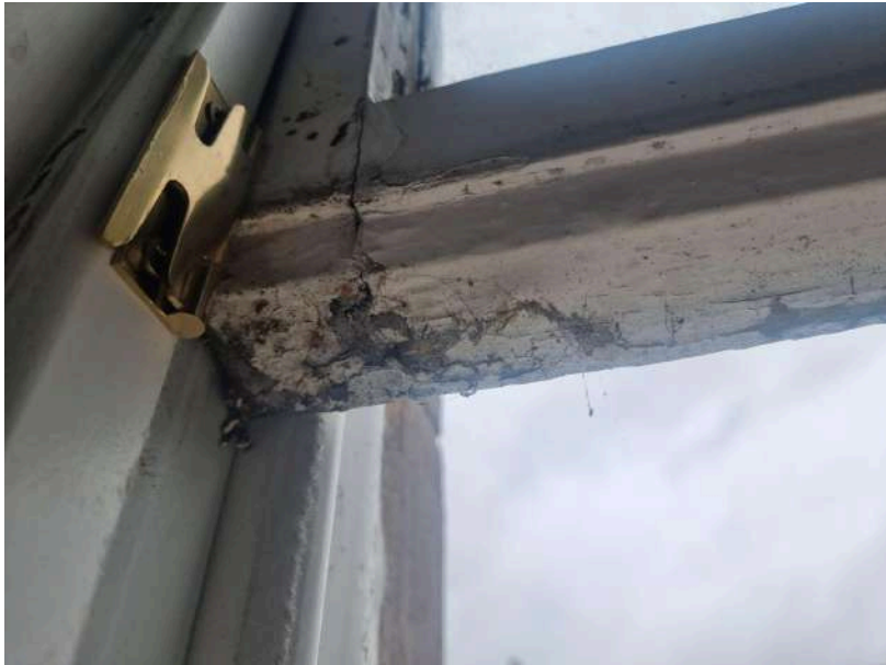
Failing tenon joint.
