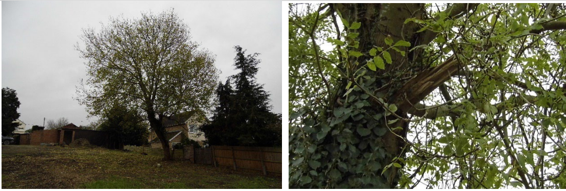
Plates 10 & 11: Views of the single ash and minor damage of one limb
