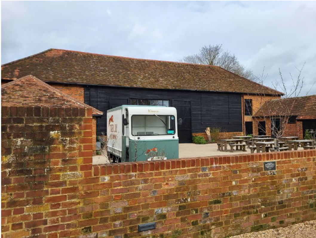
Plate 21: Southern elevation of listed five-bay former threshing barn, now converted to other uses
