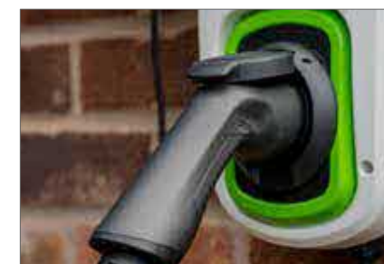
EV Charging Point
