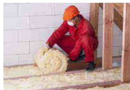
Improved Thermal Insulation
