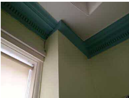
23. Switch-gear cupboard built over cornice
