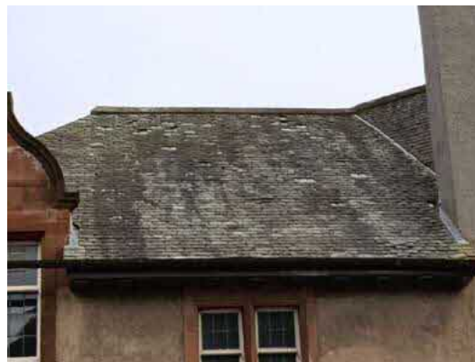
8. Defective slates to Douglas Crescent
