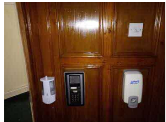
24. Surface mounted services & fittings on original hardwood panelling
