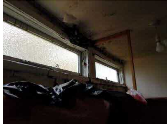
28. Evidence of moisture ingress & rot to NE extension store ceiling
