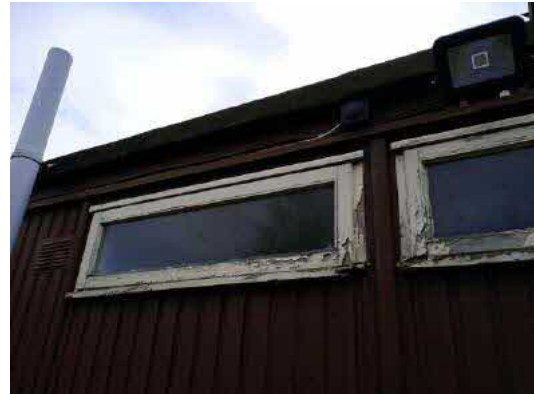
20. Rotten window frames to NE extension
