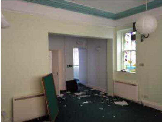
27. Evidence of previous structural slapping
