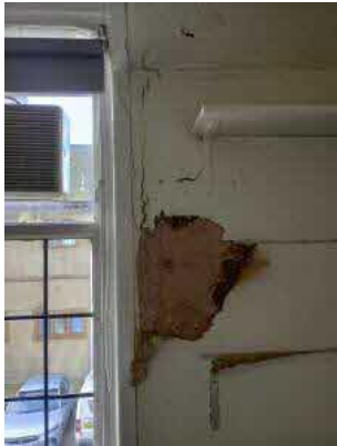
25. Dry rot to lath to side of 1 st fl window
