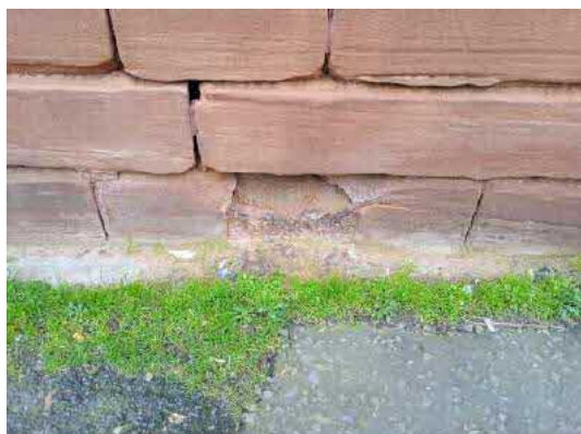
13. Salt damaged stone plinth
