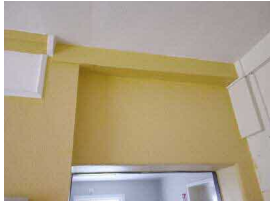
26. Evidence of previous structural slapping
