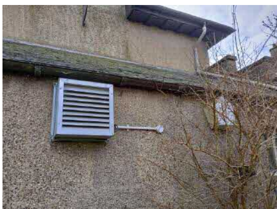
17. Surface mounted air handler to annex
