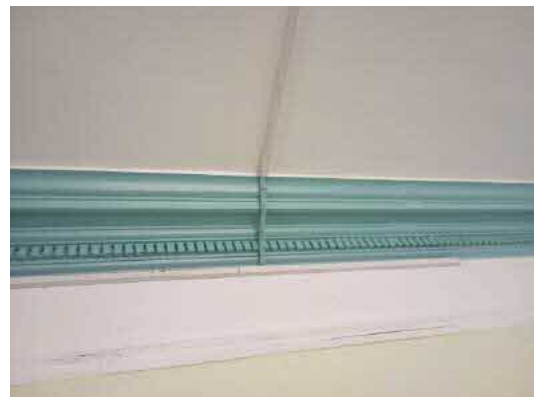
22. Surface mounted cabling over cornice
