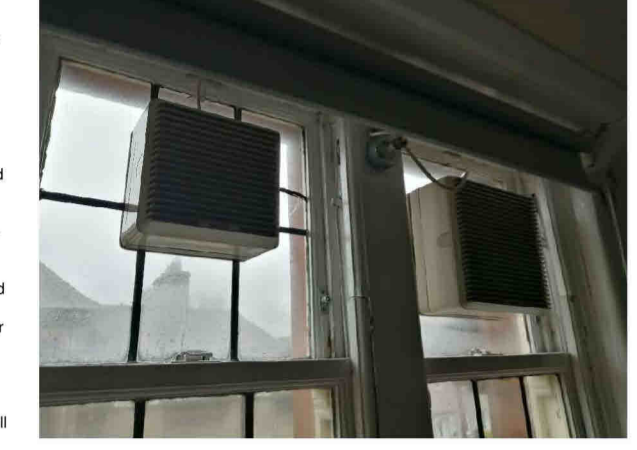
Extract Fans Cored Through Leaded Windows
