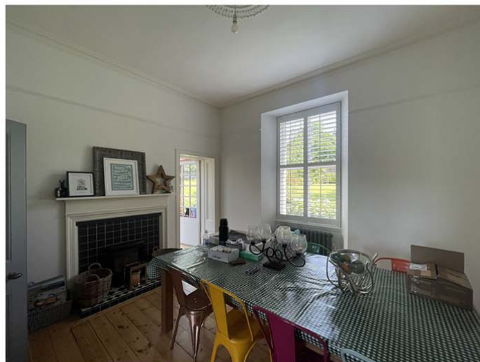
PHOTO 7. INSIDE OF EXISTING DINING ROOM WINDOW, WHERE CILL PROPOSED TO BE DROPPED.
