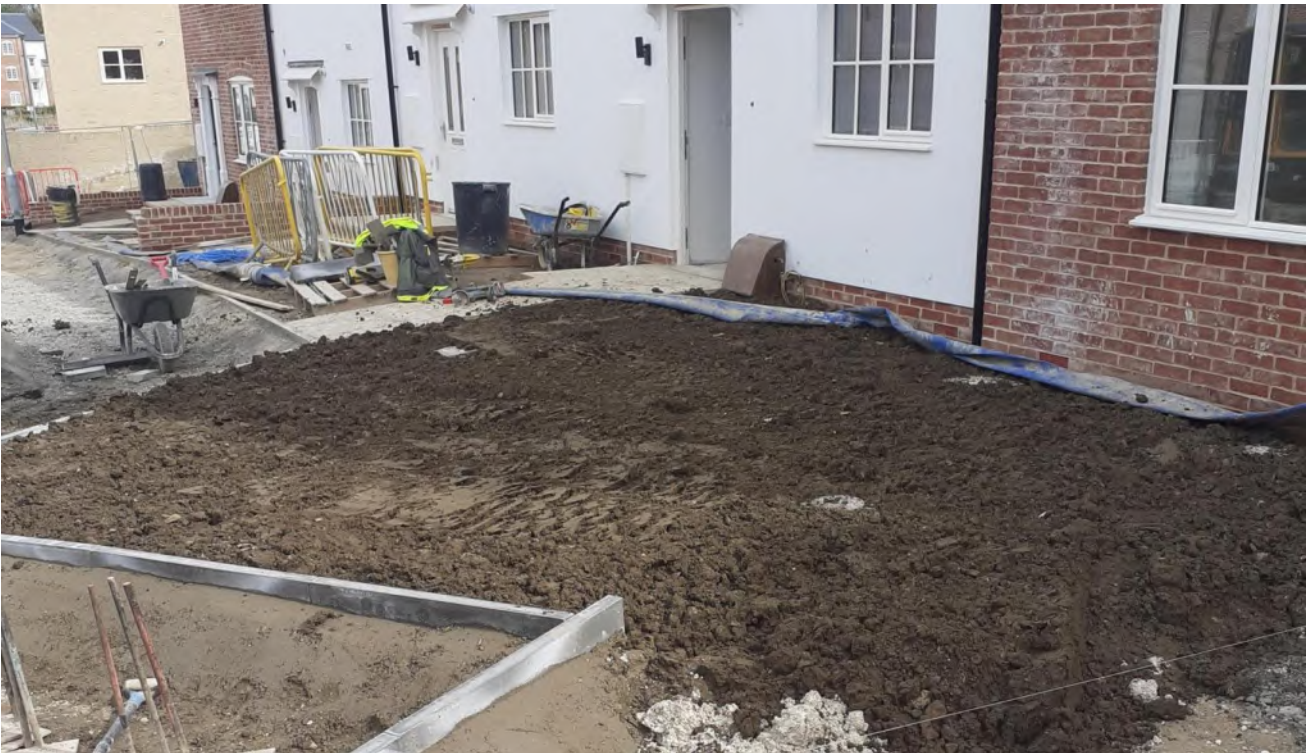
Photograph 6 , taken by the client on 12 th April 2024 showing topsoil placement within the front gardens of plots 107 and 108. Photograph taken looking towards the Southeast.
