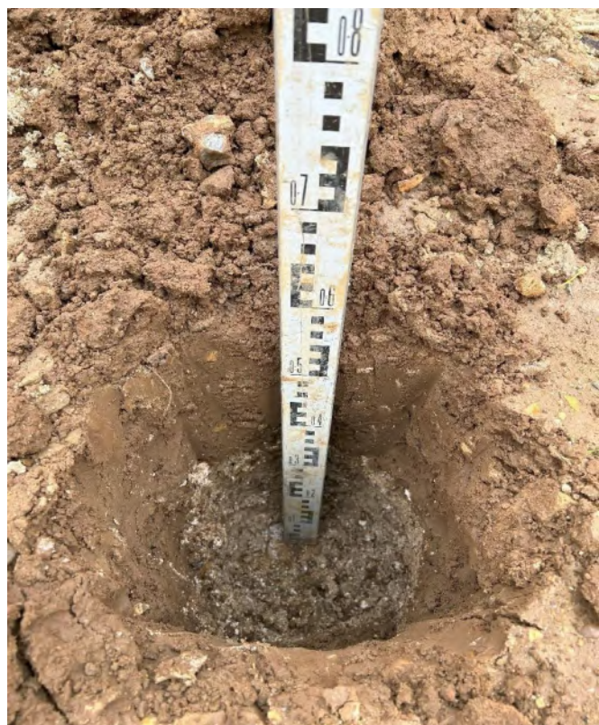
Photographs 2-3 , taken on the 20 th March 2024 showing verification hand dug trial pits in rear garden of plot 106. Photographs taken looking towards the North.
