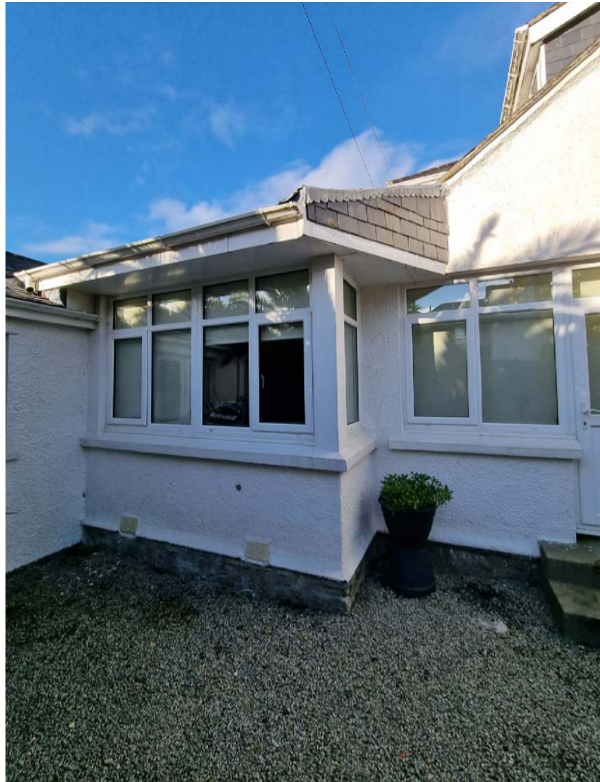
Existing poor quality U-PVC glazing to south elevation
