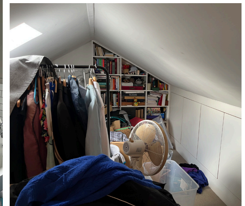
Existing non-compliant loft space
