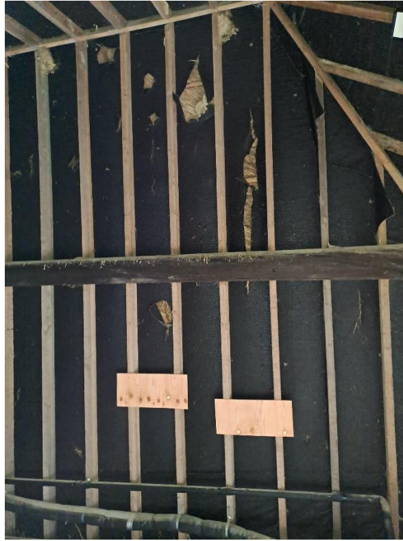
8. Torn traditional felt membrane
