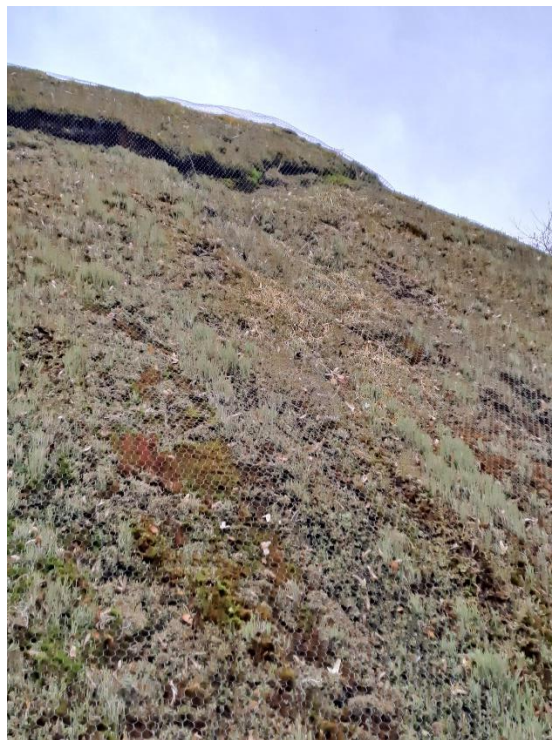
5. Close up of thatch condition
