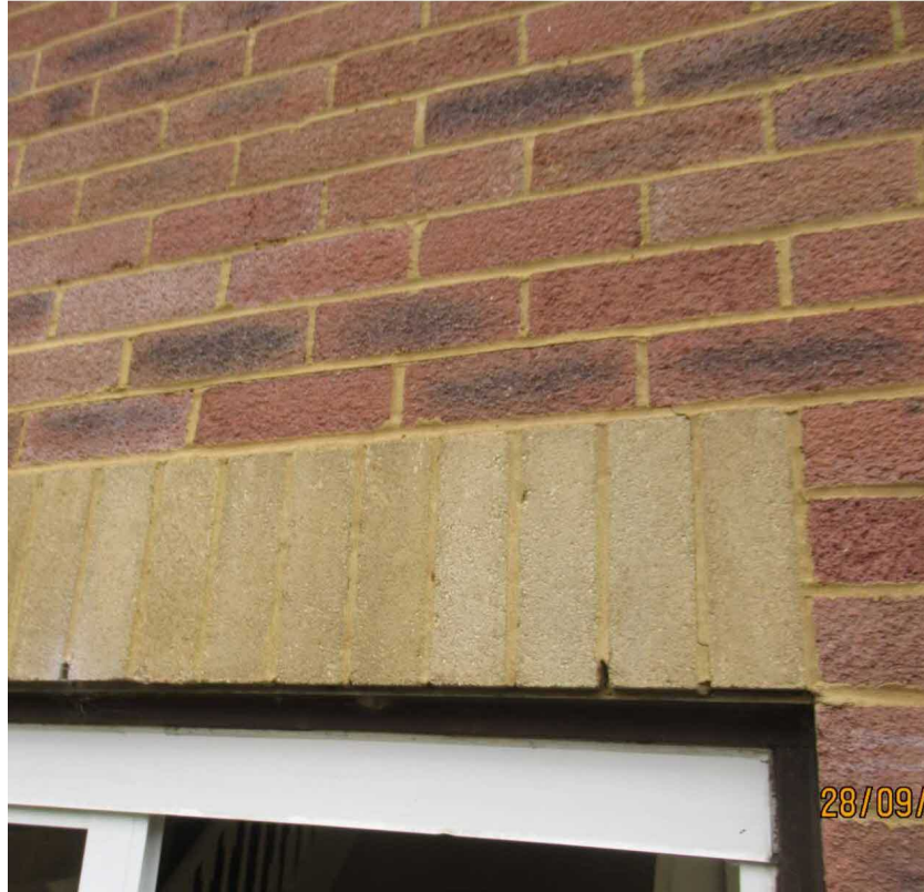
Minor cracking over patio doors
