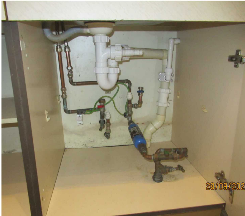
Pipework and connections underneath kitchen sink
