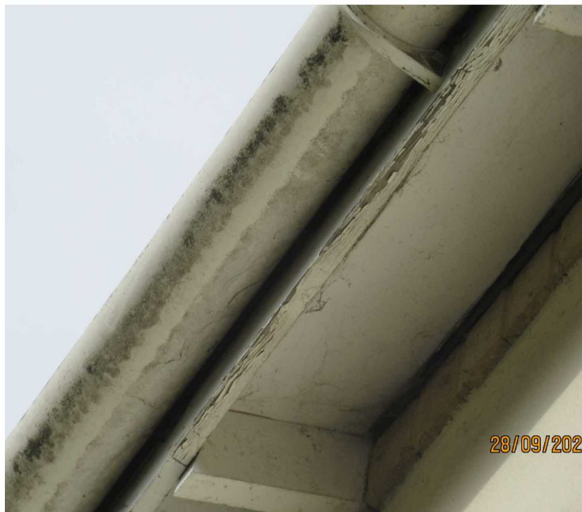
Weathered fascia to the front
