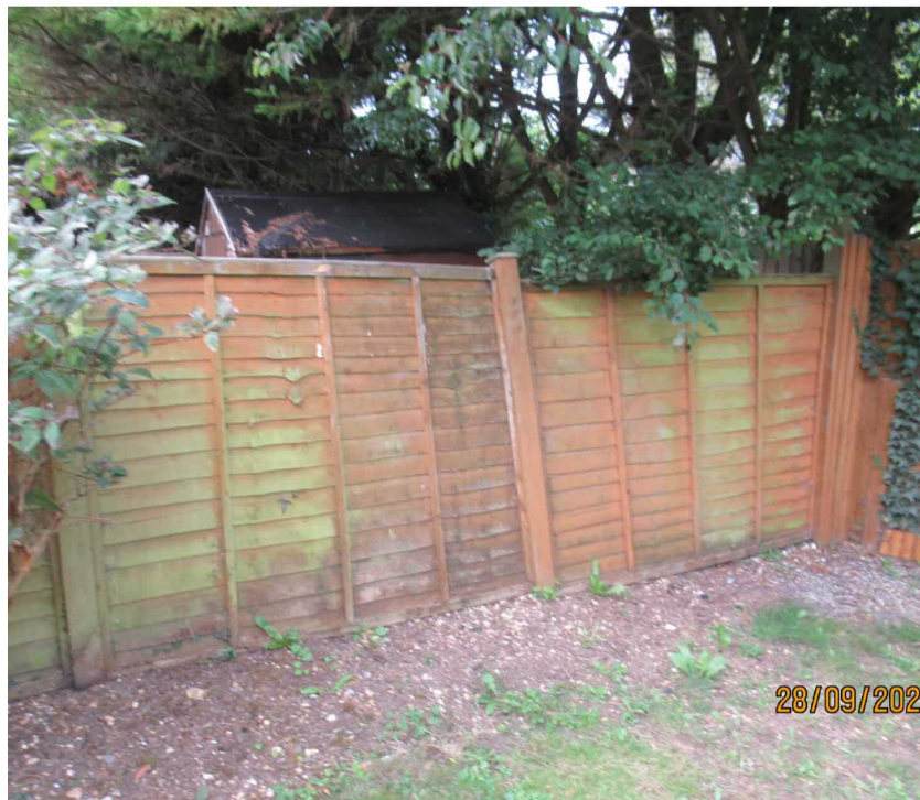
Leaning fence to rear garden
