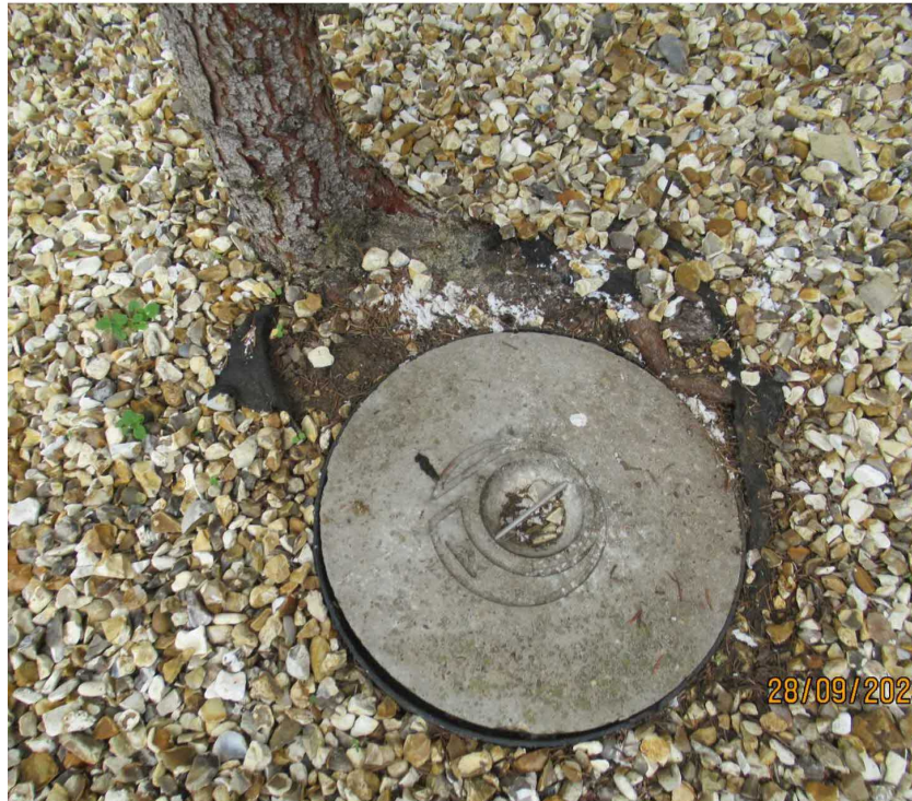
Tree roots growing around inspection chamber
