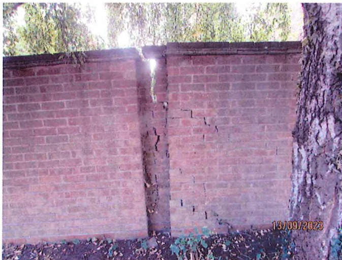
Cracked / damaged wall to front of shared parking area.
