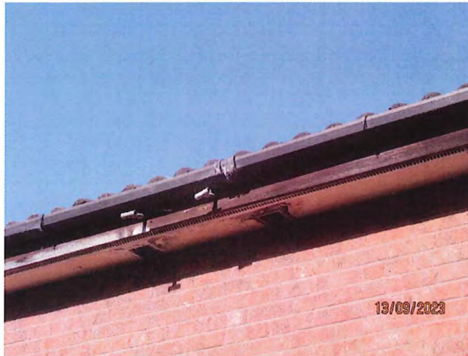
Leaking gutter joint.
