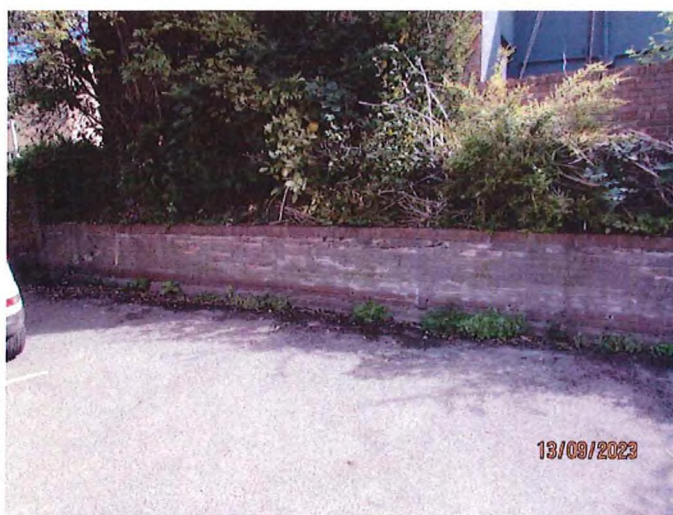
Spalled brickwork to wall to rear of shared parking area.
