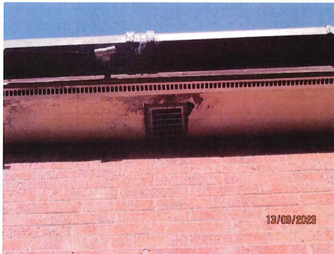
Damaged soffit board.
