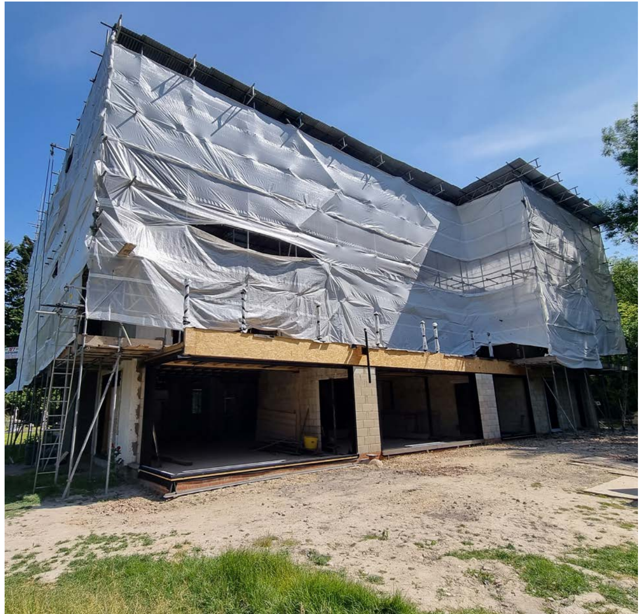
Recent site photo of the building viewed from the south west corner
