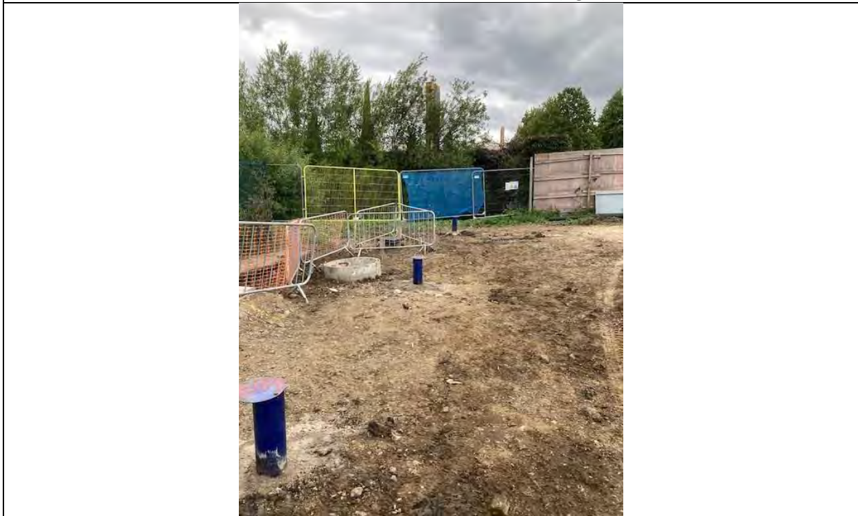
Borehole installations BH601 (foreground) 602 (middle) and BH603 (far)
