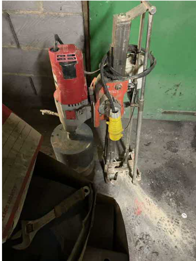
Photo 1—Example of concrete coring rig set up used to drill through concrete slab flooring in workshops
