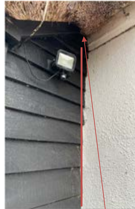
Black cable (shown here in red) to go here
