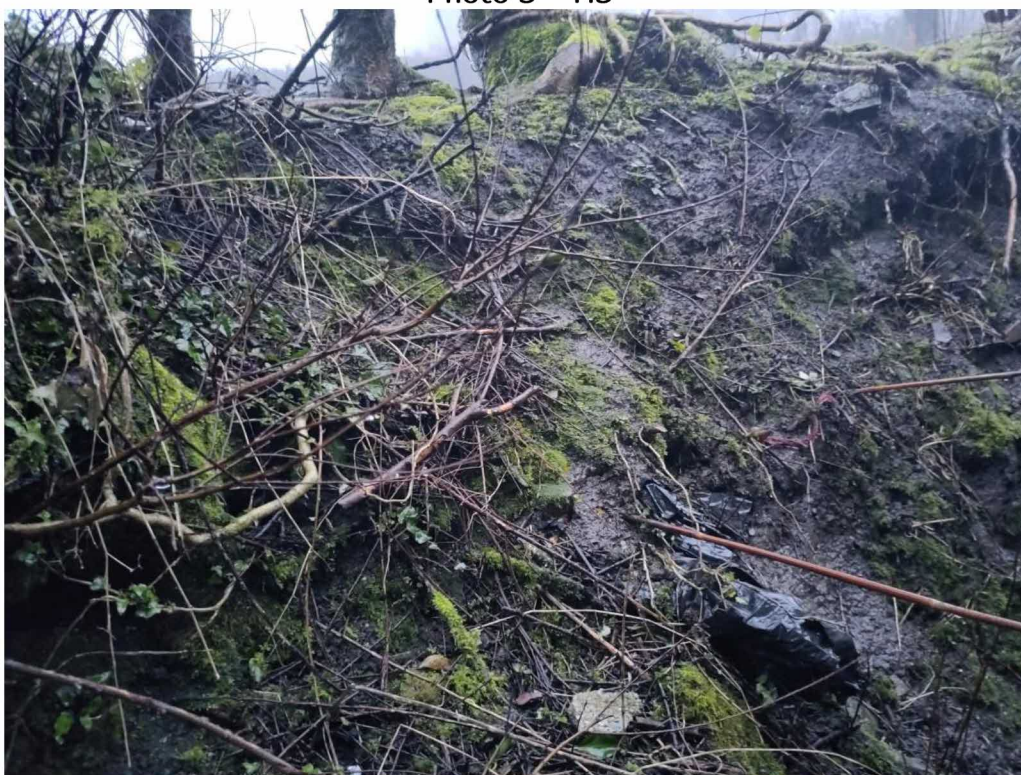
Photo 4 – H3 slumping with buried building/farm debris
