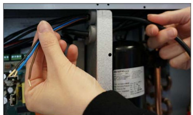
6. Run the wire from the CO 2 sensor through the cable grommet to the automation. Wire is subsequently tied up with cable strips.
