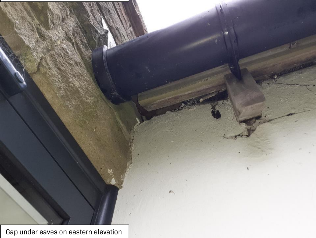
Gap under eaves on eastern elevation
