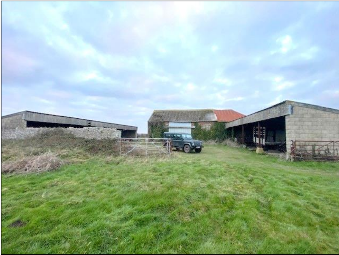
South elevation. Internal courtyard (blockwork barn to left of picture not included within application)
