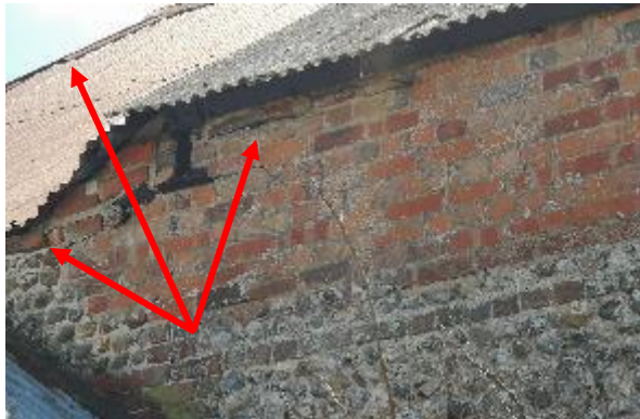
Figure 12. Gaps in the brickwork and along the hip of the roof along the northern elevation (taken June, 2022).
