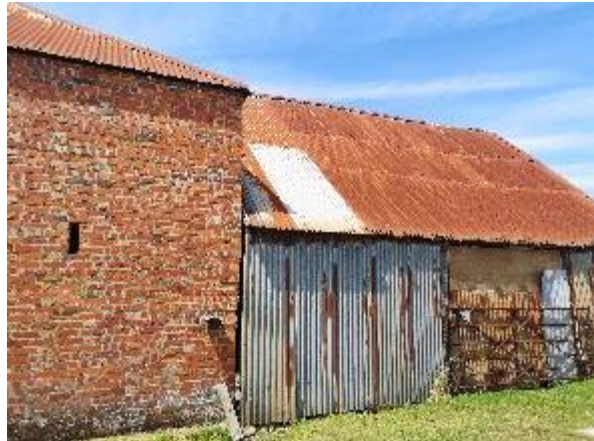
Figure 9. External view of the eastern (rear) elevation of the barn (taken June, 2022)
