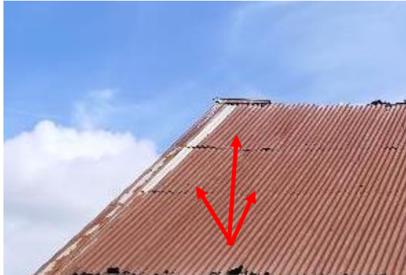
Figure 13. Gaps in the corrugated metal roofing and along the ridge on the north-western elevation (taken June, 2022)
