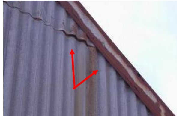
Figure 14. Slight lift and gap in the corrugated metal and along the hips on the northern elevation (taken June, 2022).
