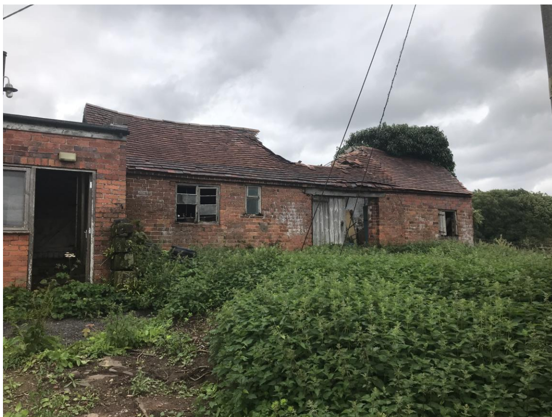
PHOTO 7 – ADJACENT OUTBUILDING WITH COLLAPSED ROOF FROM SOUTH
