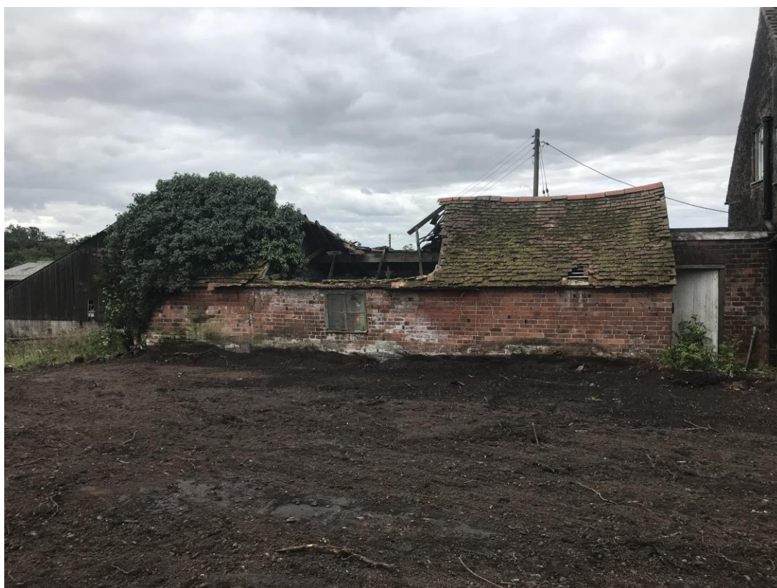
PHOTO 6 – ADJACENT OUTBUILDING WITH COLLAPSED ROOF FROM NORTH
