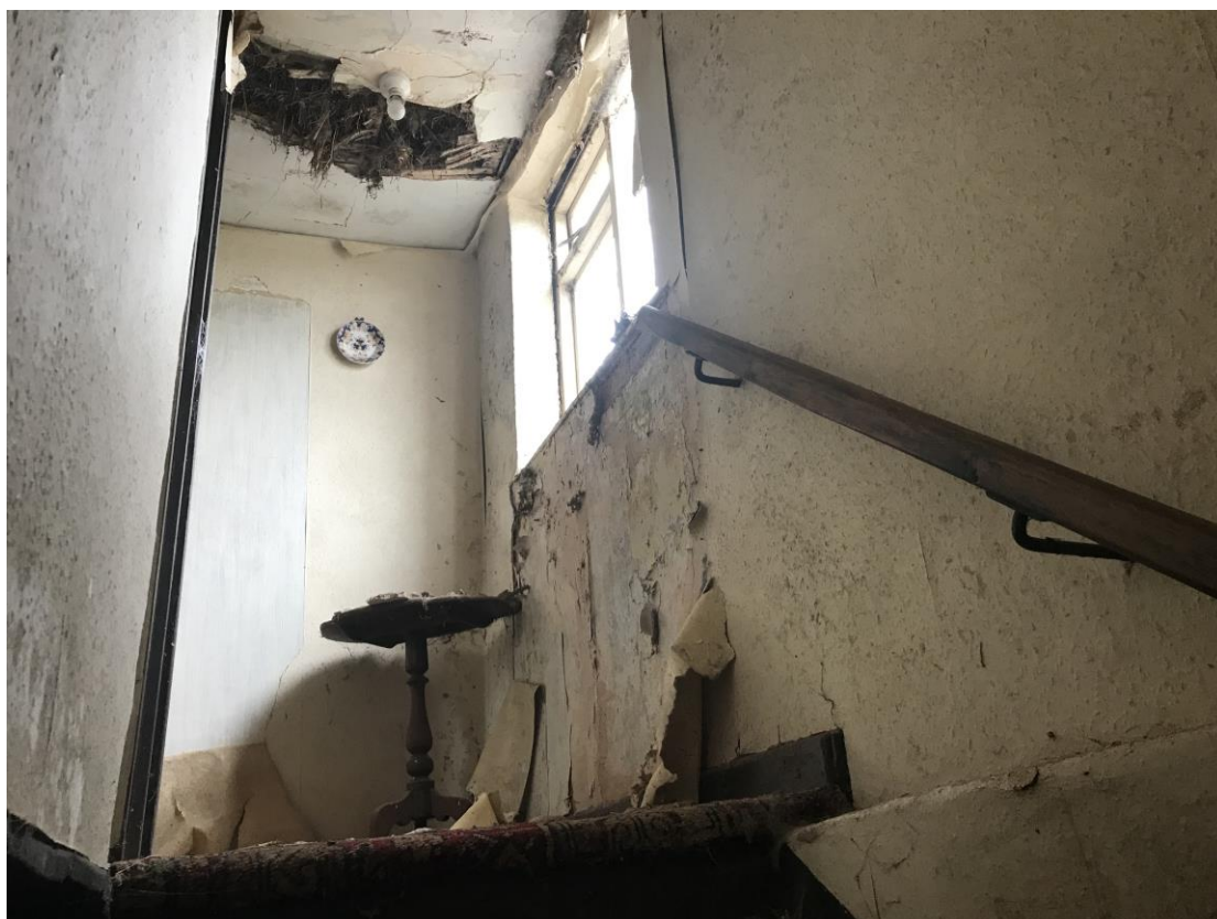
PHOTO 13 – COLLAPSED CEILING AT TOP OF STAIRS – FARMHOUSE
