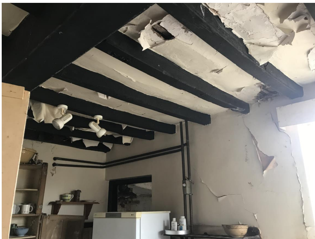
PHOTO 14 – KITCHEN WITH COLLAPSING CEILING
