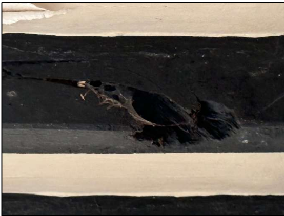
Photo 34: Missing Section of Floor Joist over Kitchen
