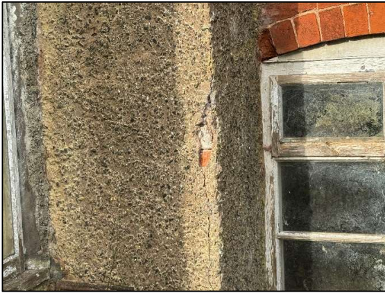
Photo 21: Crack to Render on East Elevation
