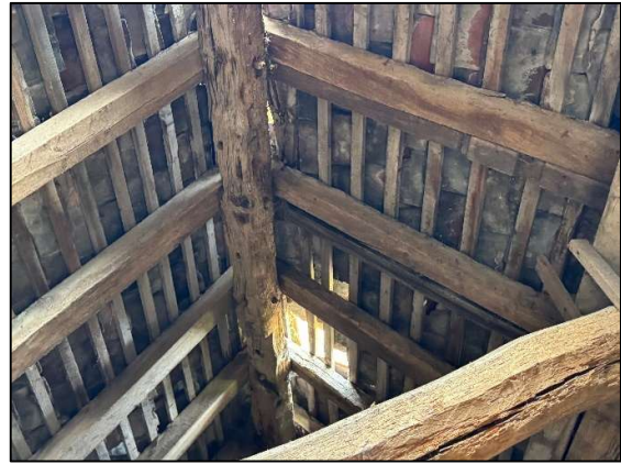
Photo 55: View of Roof Structure to Eastern End of Building with Hole in Roof
