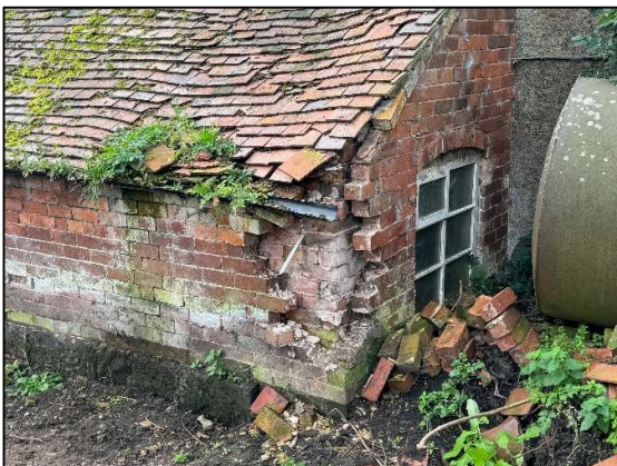
Photo 17: Damaged/Missing Brickwork to Corner of Rear Extension
