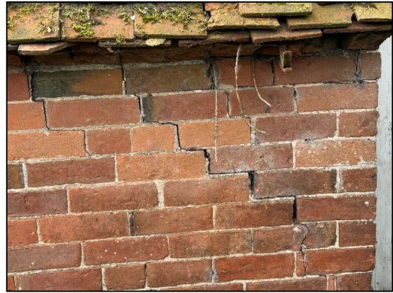
Photo 23: Crack in Brickwork on North Elevation of Barn
