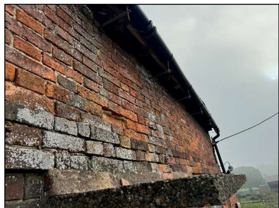
Photo 10: Spalled Brickwork at High Level
