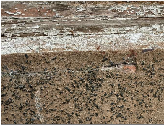
Photo 22: Crack to Render on East Elevation
