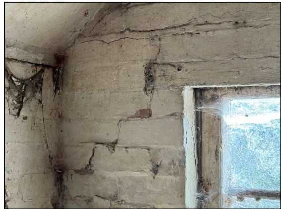
Photo 40: Cracking to Gable Wall to Rear Extension
