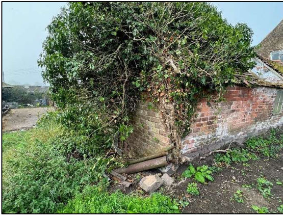
Photo 26: Tree Growing Through and Over Barn Roof
