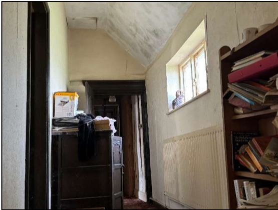
Photo 54: View of First Floor Corridor (No Safe Access Beyond This Point)
