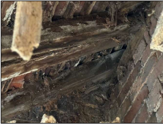
Photo 37: Decayed Roof Joists to Rear Extension
