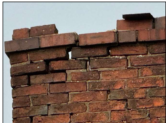
Photo 20: Loose/Displaced Brickwork to Chimney
