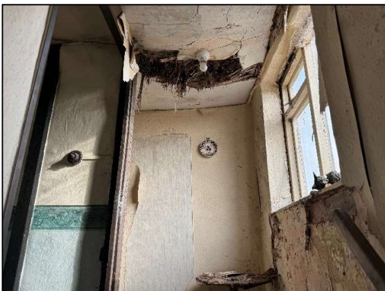
Photo 49: Partially Collapsed Ceiling at First Floor Landing
