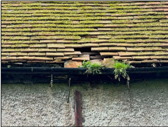
Photo 16: Missing Roof Tiles
