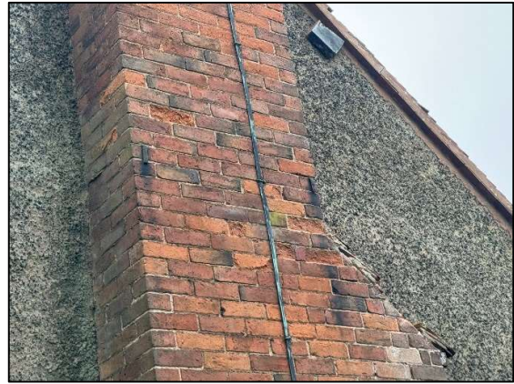
Photo 13: Spalled Brickwork to Chimney on West Elevation
