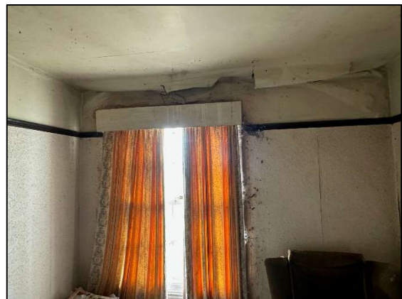
Photo 46: Damp to Front Wall and Ceiling
