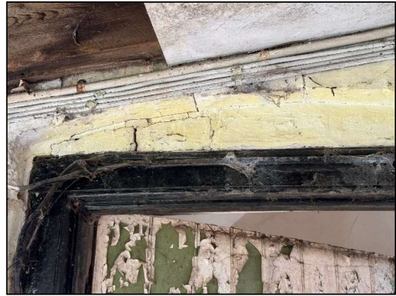
Photo 31: Cracks in Brickwork above Door Between Link Building and House
