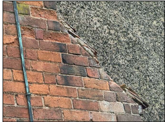
Photo 14: Missing Roof Tiles to Chimney
