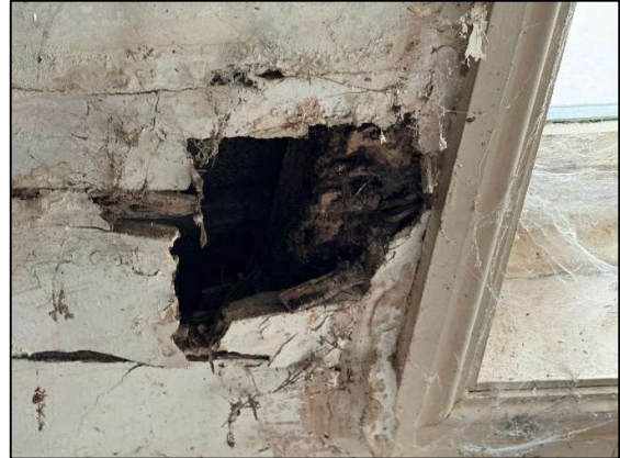
Photo 51: Decayed Ceiling/Rafter in First Floor Bedroom
