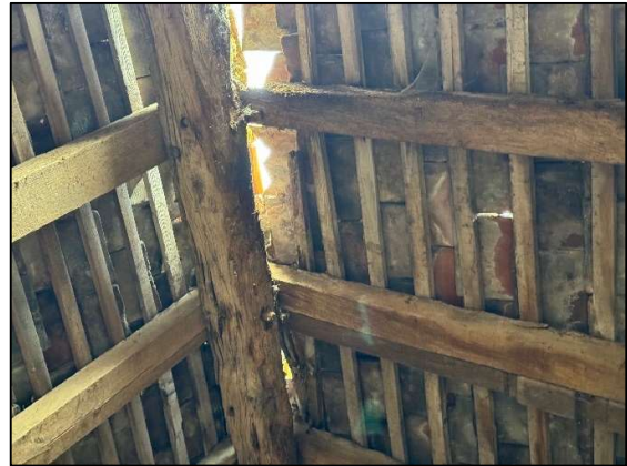
Photo 56: Holes in Roof
