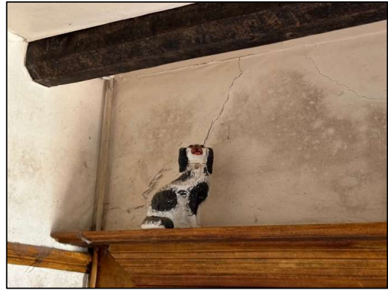
Photo 44: Crack in Wall above Fireplace
