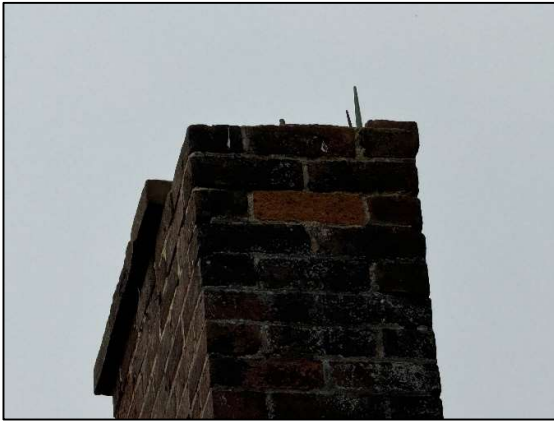
Photo 15: Missing Bricks to Top of Chimney
