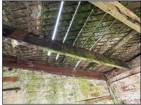
Photo 28: Gaps in Link Building Roof with Missing Felt
