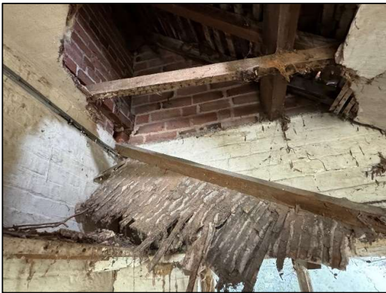
Photo 38: Collapsed Ceiling Joist to Rear Extension
