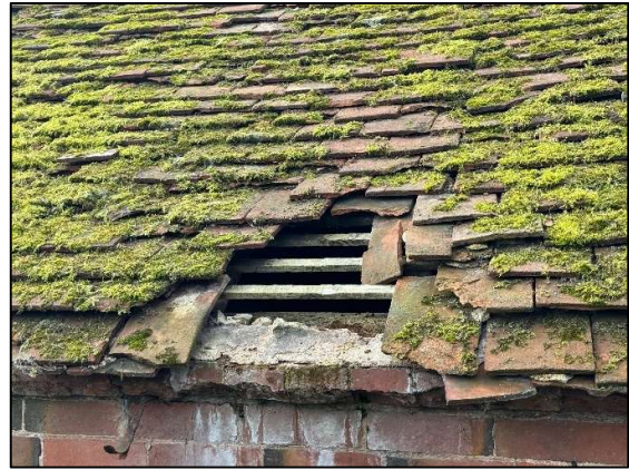
Photo 24: Missing Roof Tiles to Barn Roof
