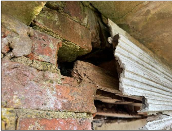
Photo 11: Decayed Timber Lintel over Front Door
