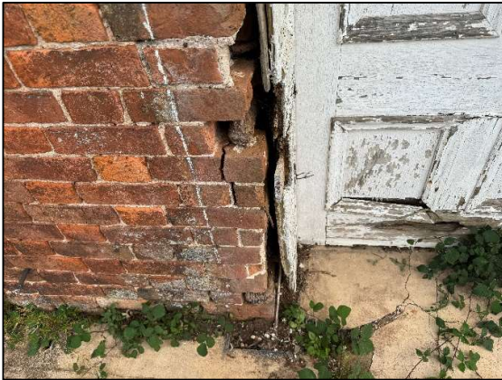
Photo 12: Cracked/Missing Brickwork to Side of Front Door
