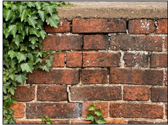
Photo 8: Cracking in Brickwork Beneath Ground Floor Window
