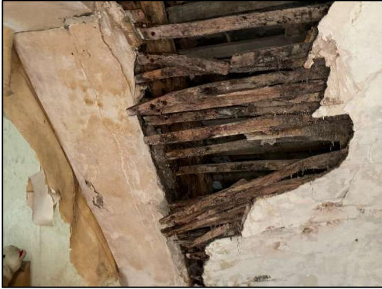
Photo 57: Decayed Ceiling at First Floor Level
