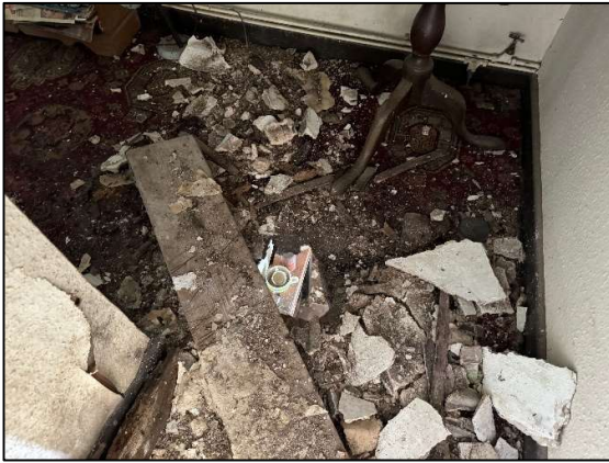
Photo 53: Hole in Floorboards in First Floor Corridor
