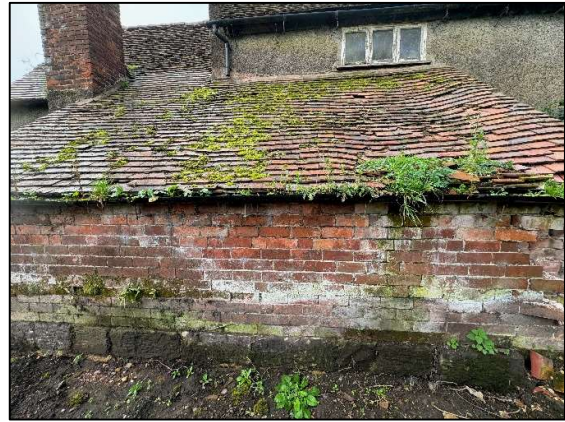
Photo 18: Uneven Roof to Rear Extension
