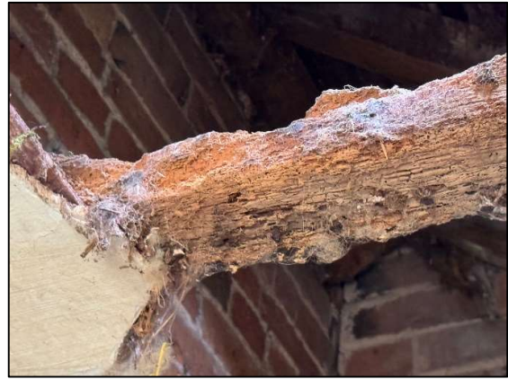
Photo 39: Decayed Ceiling Joist to Rear Extension
