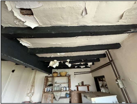
Photo 33: View of Damp to Kitchen Ceiling
