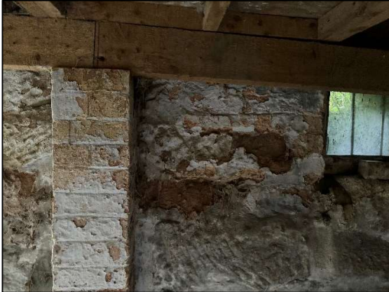
Photo 48: Spalled Brickwork to External Wall to Basement
