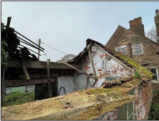
Photo 25: Collapsed Roof to Barn and Leaning Side Wall
