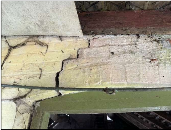
Photo 30: Cracks in Brick Arch above Door between Link Building and Barn
