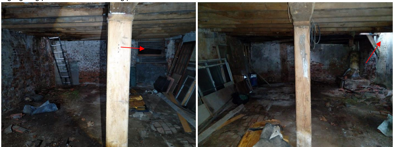
Plate 4.5 – (L) – Internal of room 2, ground floor, facing West, (R) – Internal of room 2, ground floor, facing East; highlighting potential access/roosting points
