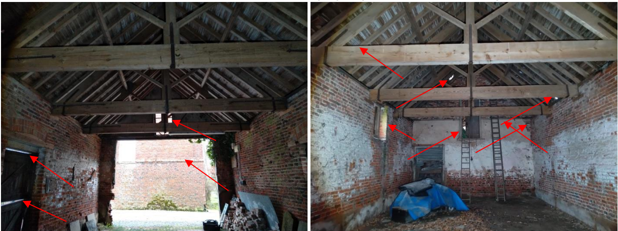
Plate 4.3 – (L) – Internal of room 1, facing south (R) – Internal of room 1, facing north; highlighting potential access/roosting points
