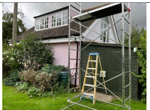
Photo 6. Rear and east elevations of garage showing roof tiles and soffits in good condition
