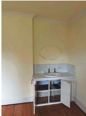
Alcove in master bedroom through which en suite bathroom doorway to be formed.
