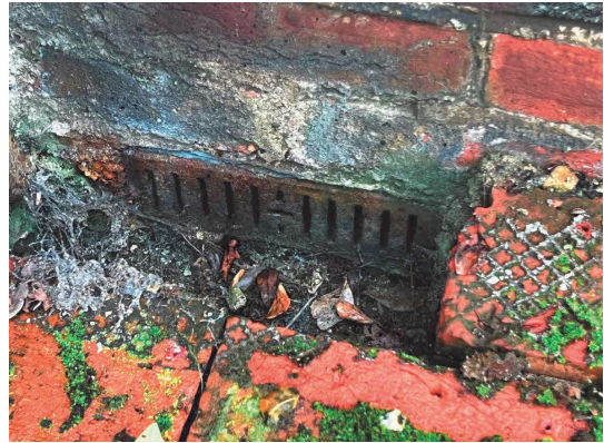
'Existing cast iron air brick detail (maintained with surrounding brick due to raised external ground level).
