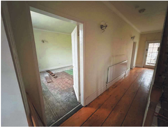
View showing section of wall, door set and skirting proposed to be removed and relocated.
