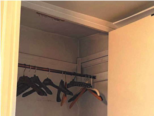
Remnants of original picture rail proposed to be reinstated throughout the house.
