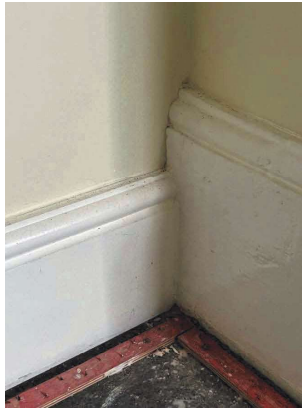
Modern skirting board (left) proposed to be replaced with match for original skirting (right).
