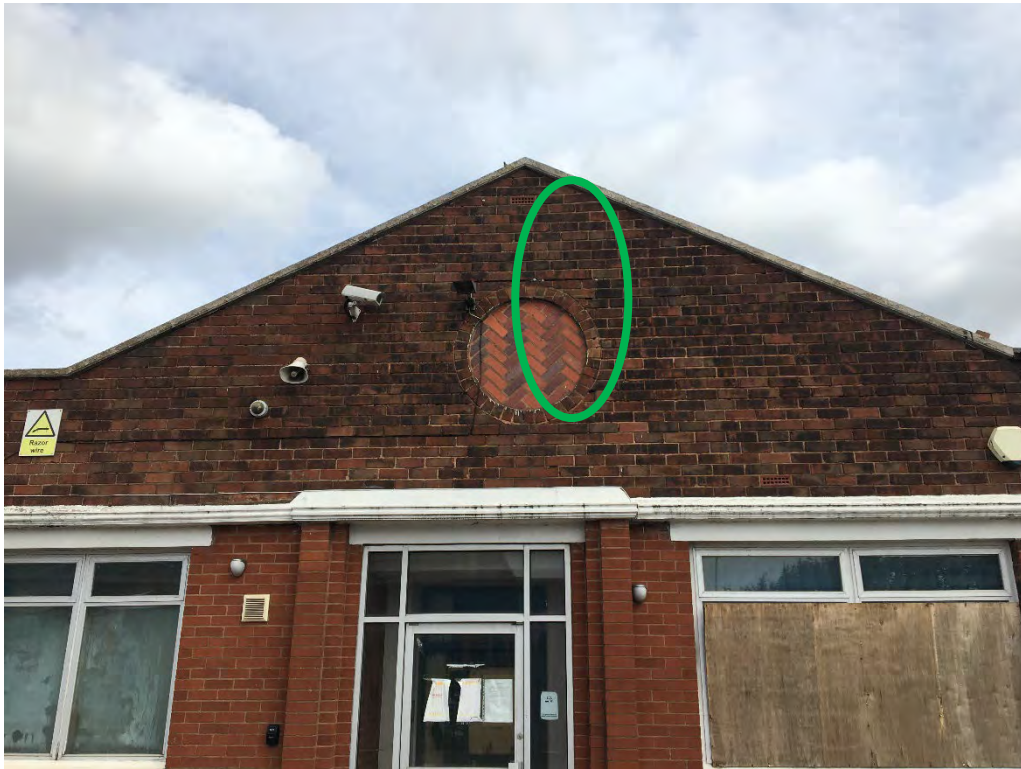
Photograph 5 - Potential bat roost feature identified on the building (TN 1)
