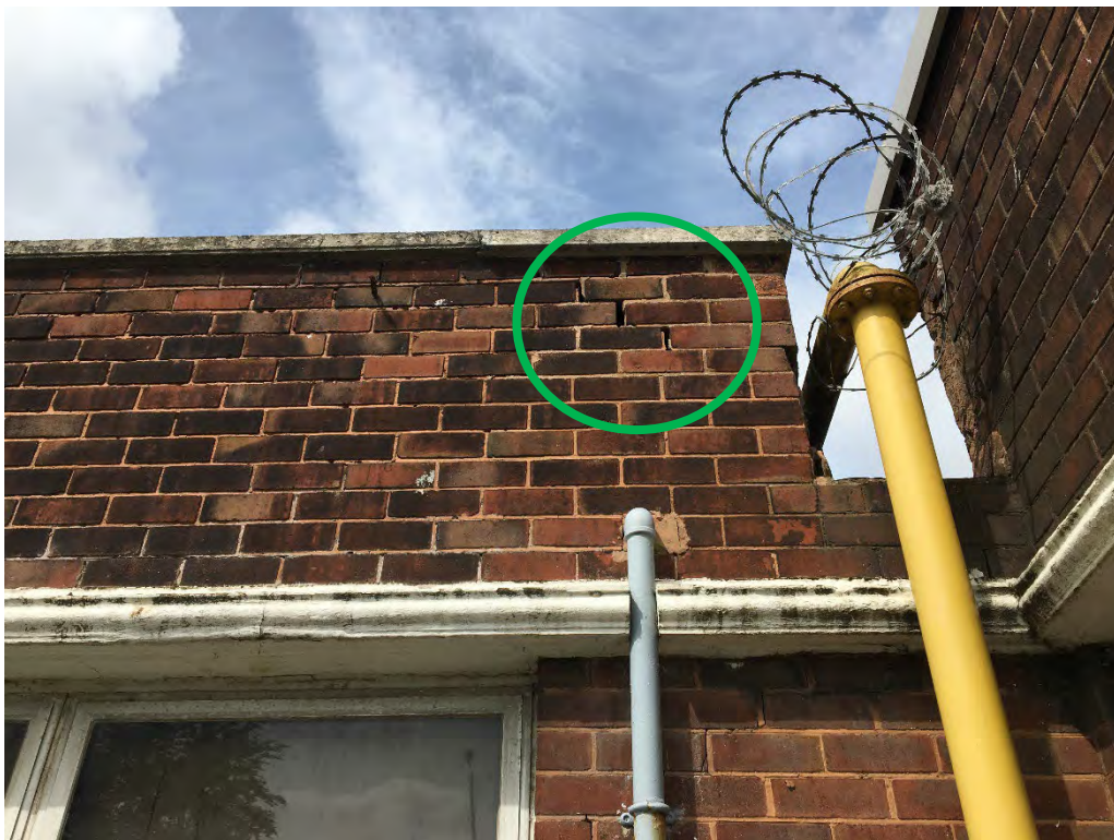
Photograph 6 - Potential bat roost feature identified on the building (TN 2)
