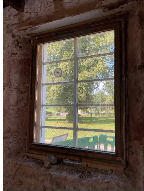
Internal view of GW02 (note: inner window is a reclaimed window installed backwards)
