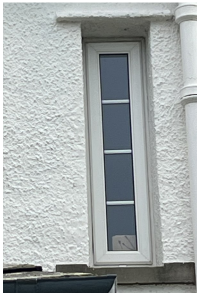
No. 24 - PVC Signs of double glazing failing causing internal condensation, loose internal astragals and inappropriate existing material.
