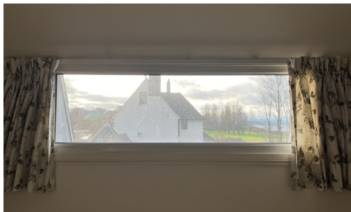
No. 21 & 27 - PVC Signs of double glazing failing causing internal condensation, loose internal astragals and inappropriate existing material.
