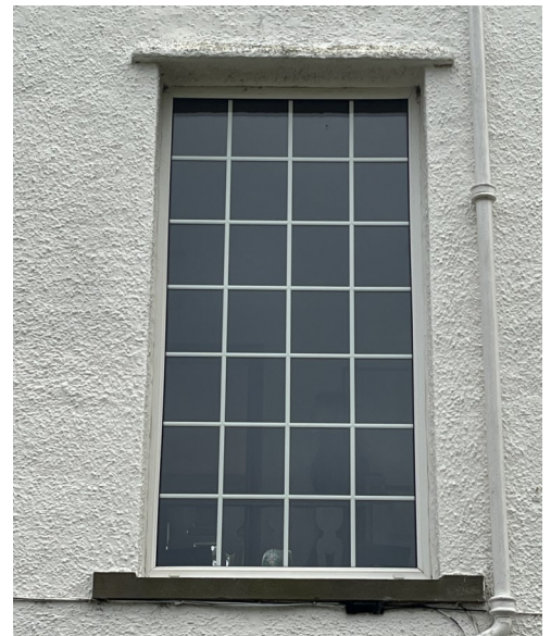
No. 25 - PVC Signs of double glazing failing causing internal condensation, loose internal astragals and inappropriate existing material.
