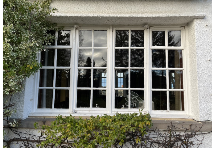
No. 02 - Existing Steel Crittall Style Windows are drafty, deteriorating, rusting beyond repair and not functional due to failure to open causing lack of ventilation. Additionally window panels are cracked due to ageing and weathering.
