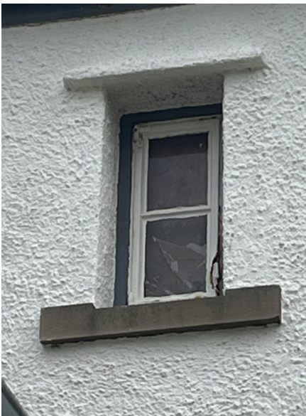
No. 23 - Existing Steel Crittall Style Boarded up window due to extreme damage and crack to the glazing.
