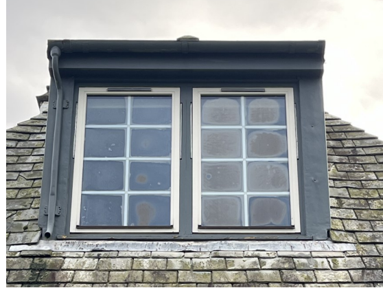
No. 22 - PVC Double glazing failing causing internal condensation between panels, loose internal astragals and inappropriate existing material.
