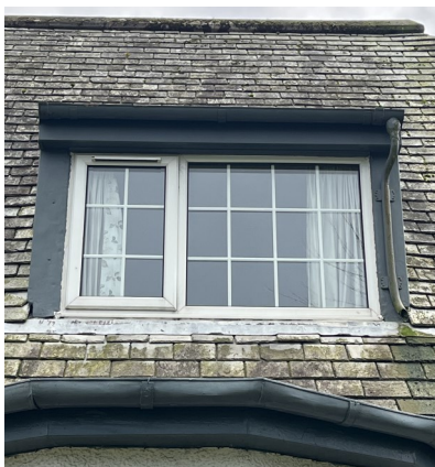
No. 26 - PVC Signs of double glazing failing causing internal condensation, loose internal astragals and inappropriate existing material.
