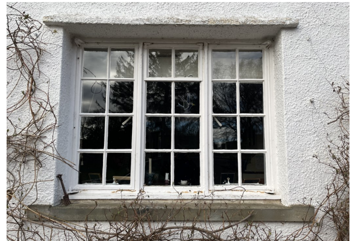
No. 04 - Existing Steel Crittall Style Windows are drafty, deteriorating, rusting beyond repair and not functional due to failure to open causing lack of ventilation.
