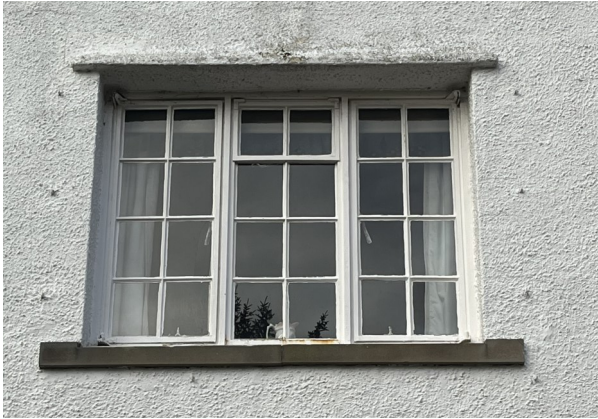
No. 20 - Existing Steel Crittall Style Windows are drafty, deteriorating, rusting and not functional due to failure to open causing lack of ventilation. Additionally window panels are cracked due to ageing and weathering.
