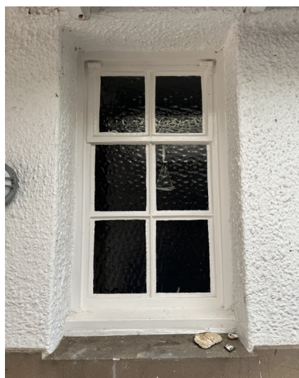
No. 06 - Existing Steel Crittall Style Windows are drafty, deteriorating, and not functional due to failure to open causing lack of ventilation.
