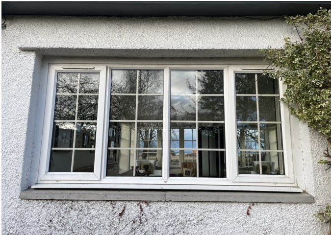
No. 01 - PVC Signs of double glazing failing causing internal condensation, loose internal astragals and inappropriate existing material.
