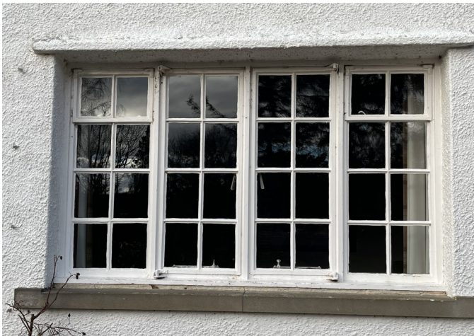
No. 03 - Existing Steel Crittall Style Windows are drafty, deteriorating, rusting beyond repair and not functional due to failure to open causing lack of ventilation.
