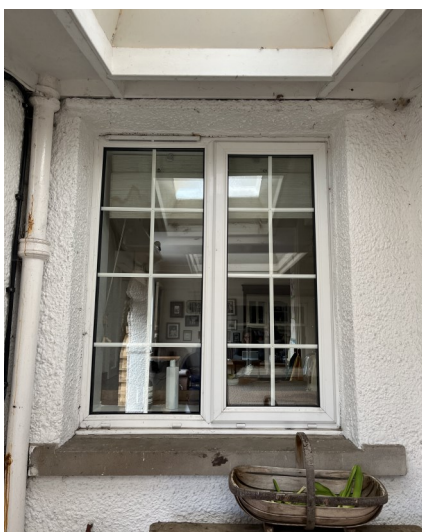
No. 05 - PVC Signs of internal condensation, loose internal astragals and inappropriate existing material.
