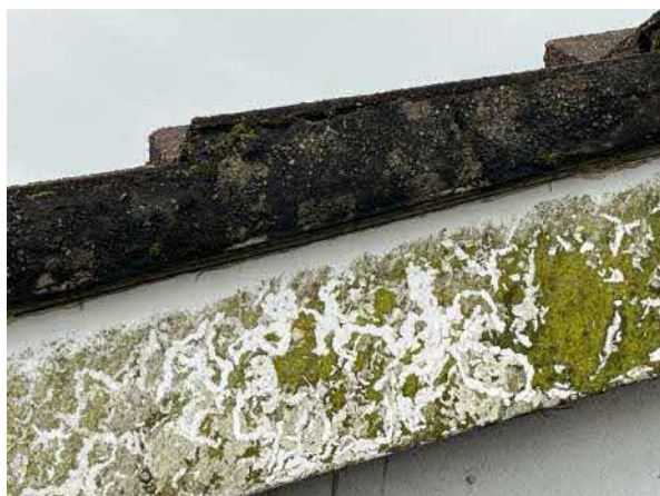
Photograph 8. Cement seal at gable end of tiles.
