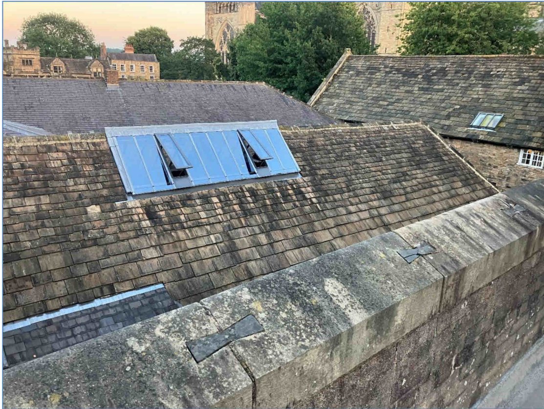
Photograph 3 – West elevation of Palace Green library roof viewed from roof of adjacent building
