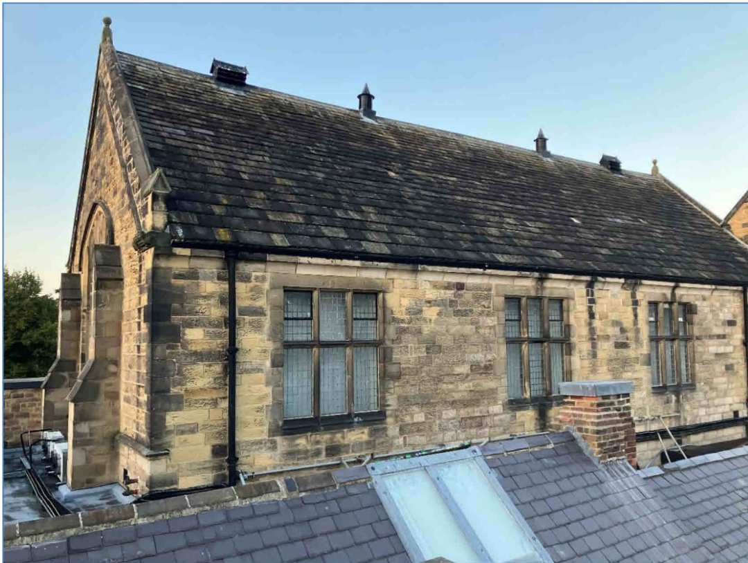
Photograph 2 – South and West elevations of The Education and Learning Centre viewed from roof of neighbouring building.
