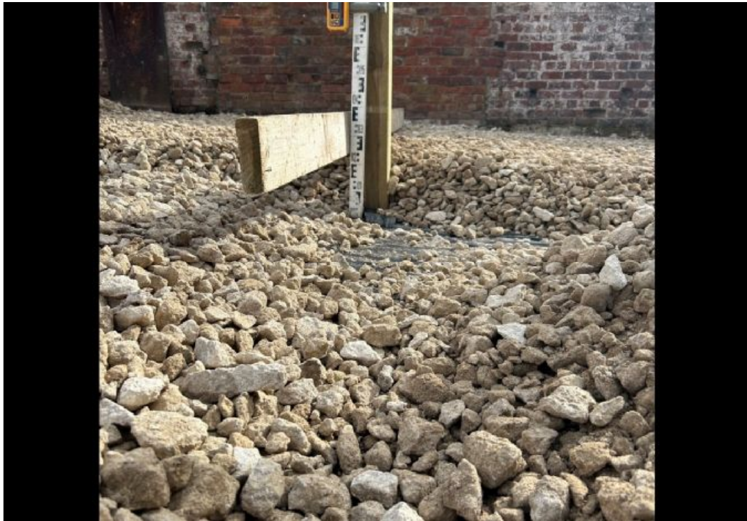
Evidence of level control
