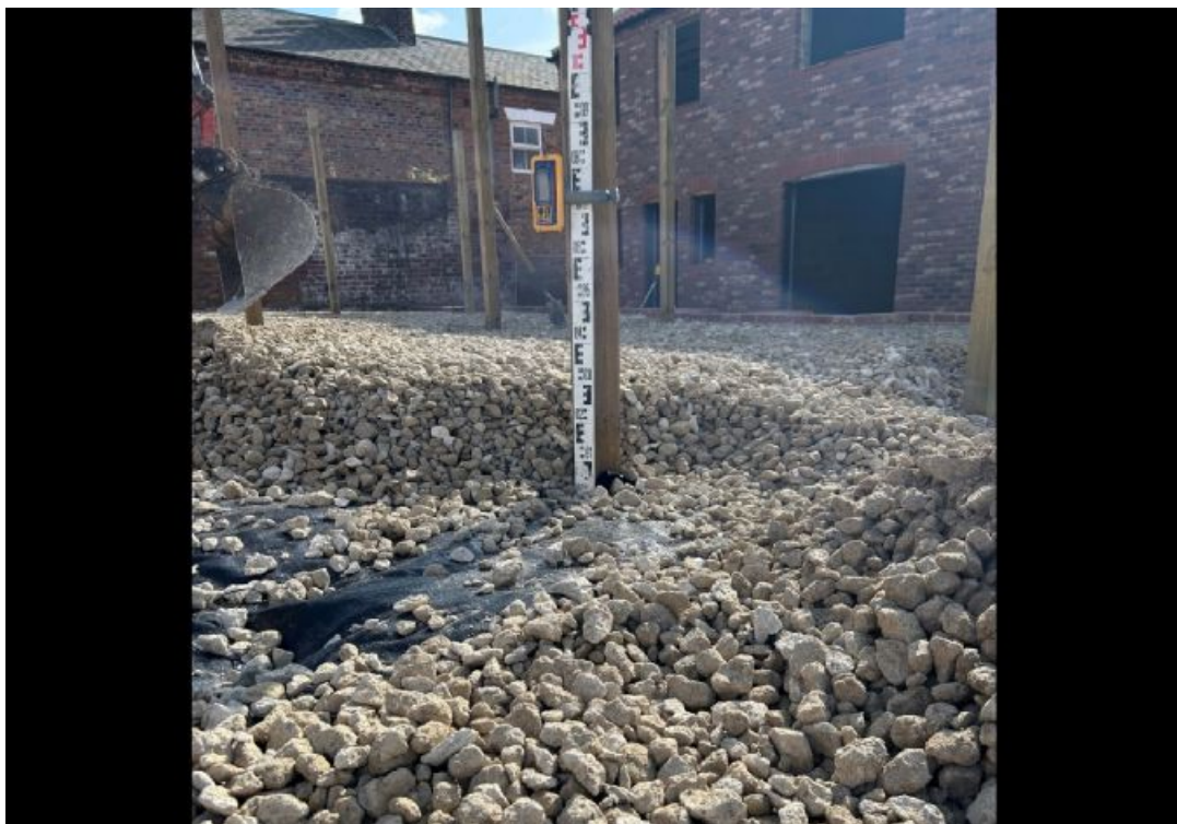
Evidence of level control
