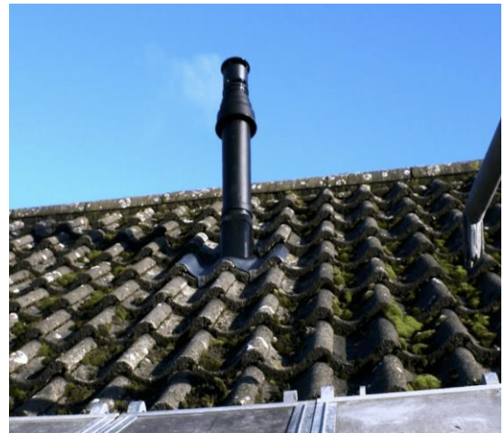
Black coated boiler flue: Utility Roof
