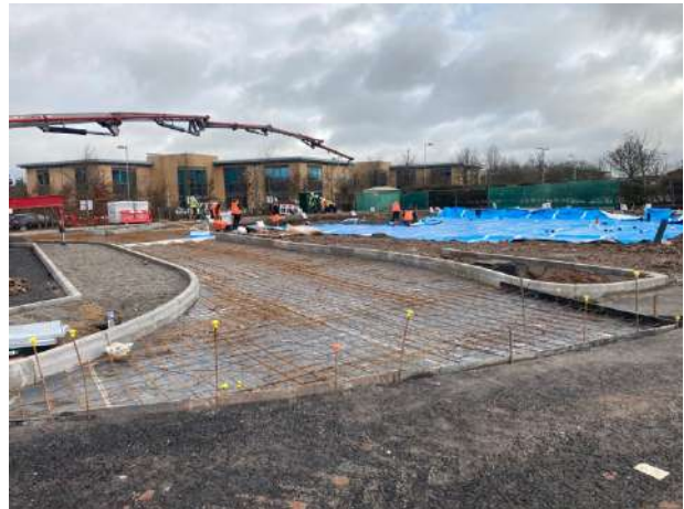
Photo 10: Access road around McDonalds unit in the process of receiving concrete on 16 th February 2024.
