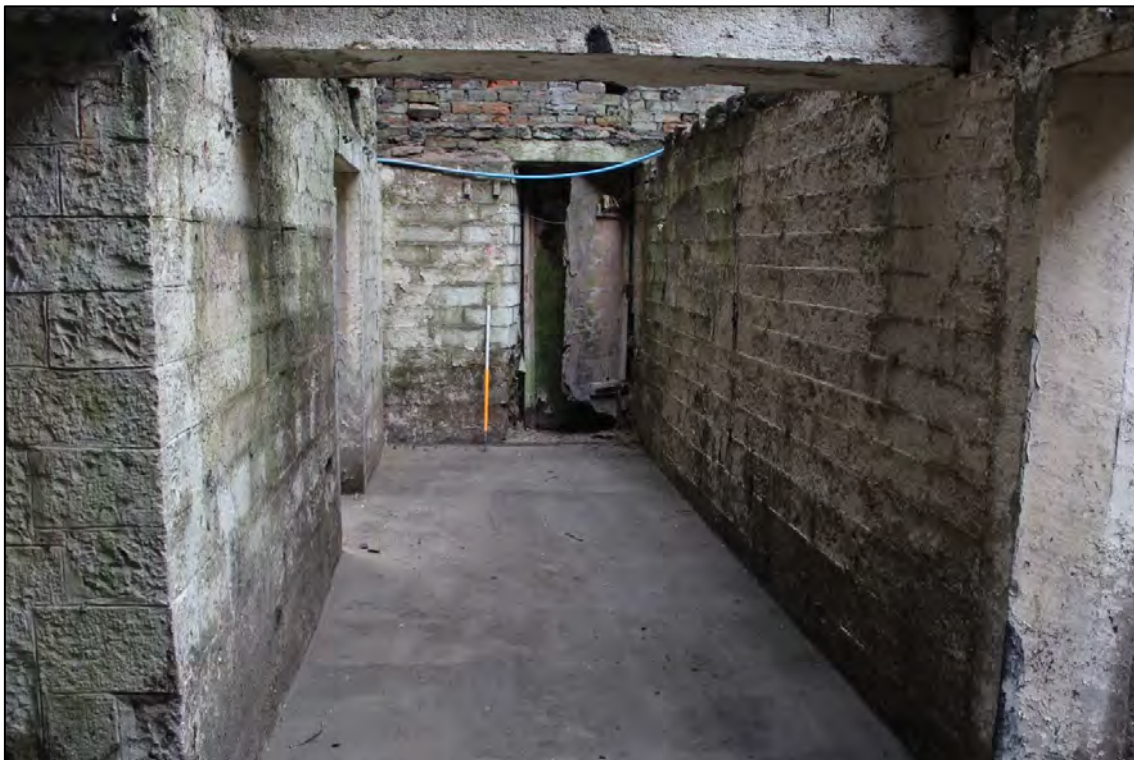
Plate 16: Internal view looking S within the basement corridor towards the external entrance to the S
