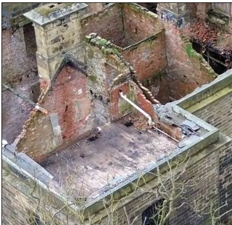
Plate 90: View looking SE towards two inaccessible first floor and attic level compartments
