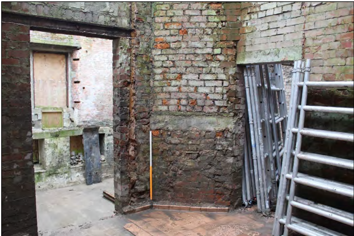
Plate 58: Internal view looking SE within a ground floor service compartment
