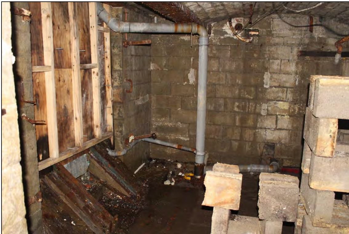
Plate 15: Internal view looking SSE towards the western external entrance within the basement
