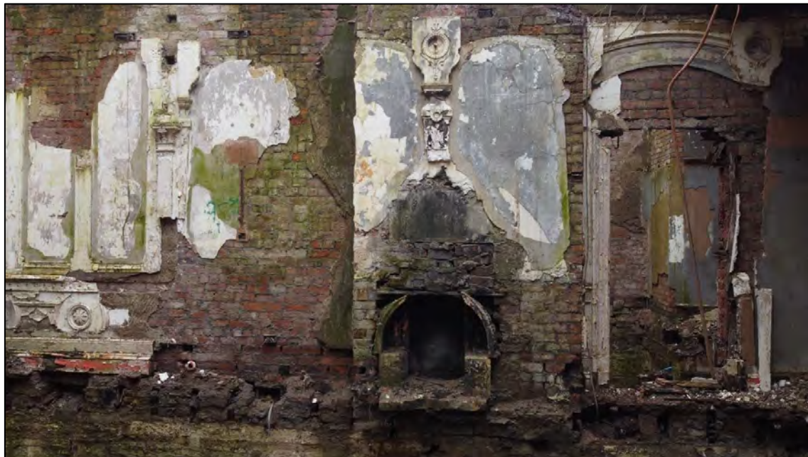
Plate 63: internal view looking S showing the wall mouldings at ground floor level within the entrance hall
