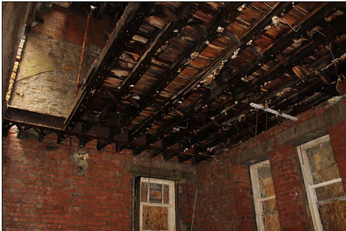
Plate 67: internal view looking NW at the only surviving ceiling at ground floor level
