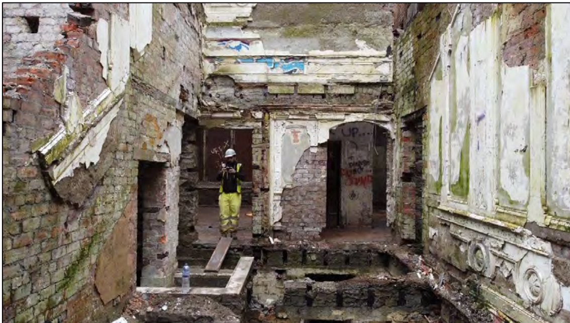
Plate 35: Internal view looking E along the entrance hall at ground floor level
