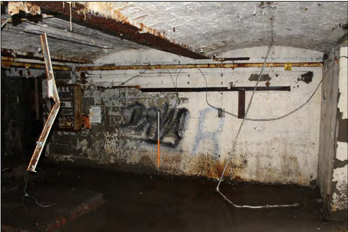
Plate 27: Internal view looking SSW showing the vaulted brick ceilings within the basement
