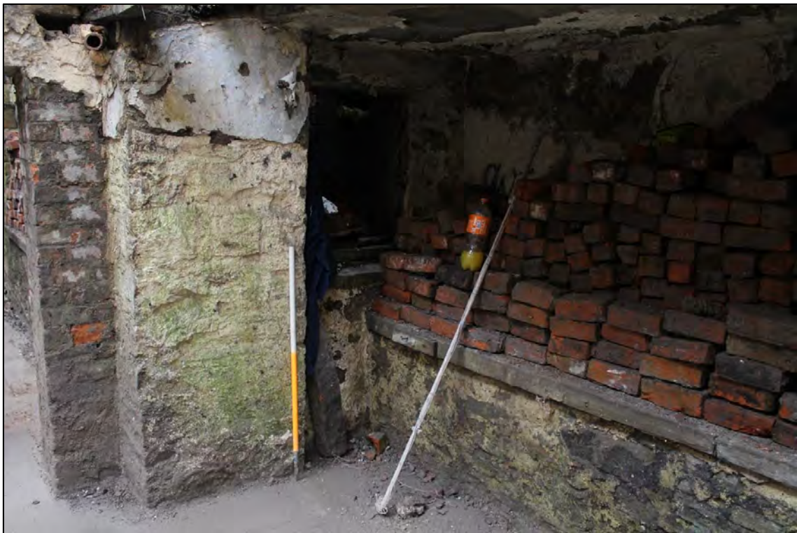
Plate 19: Internal view looking SW within the western end of the central corridor within the basement
