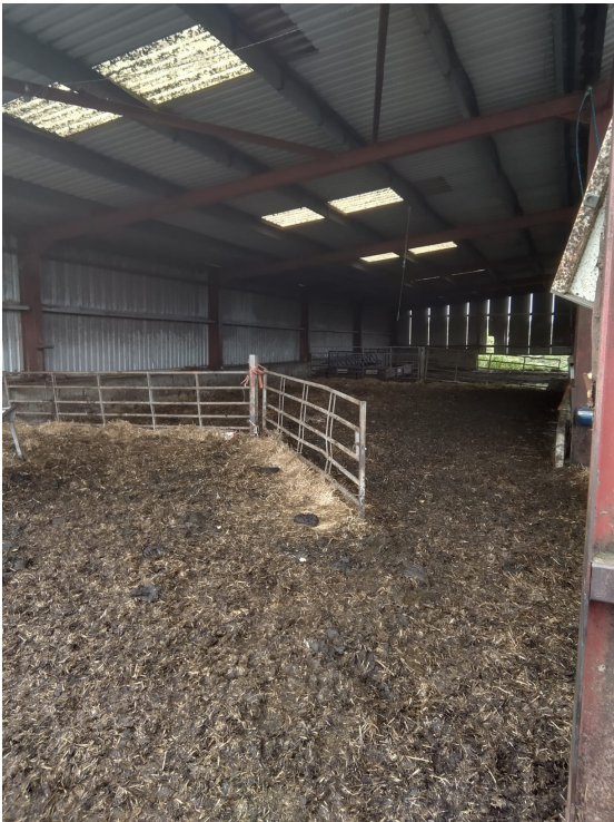
Internal images of the existing shed, showing the existing steel portal frame in good condition, and suitable for conversion.
