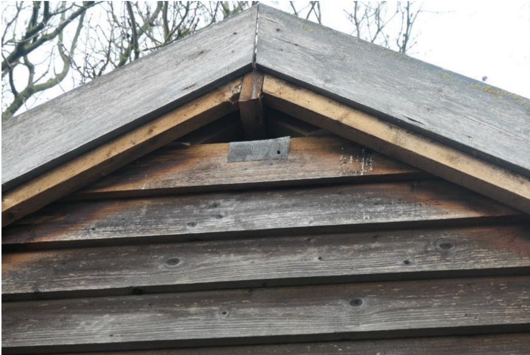
Photo 8 , gap at the apex of the southern aspect allowing access into the small, closed void.
