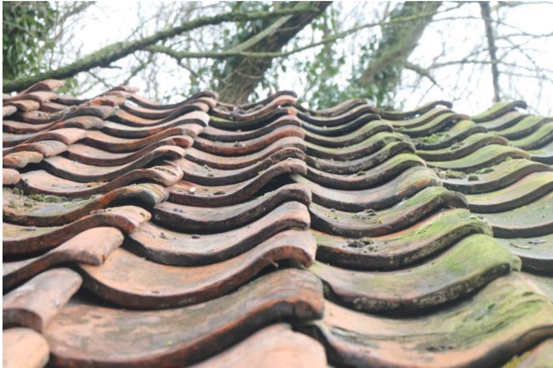
Photo 10 , gaps under tiles on the western aspect and missing ridge tiles.
