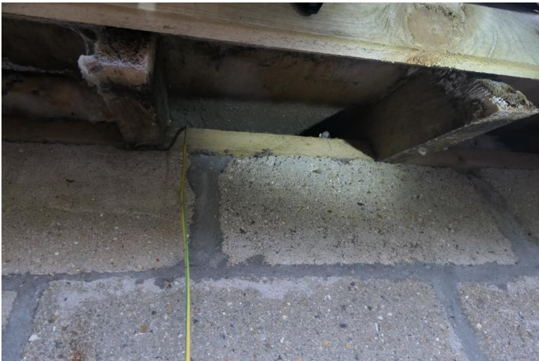
Photo 9 , gaps at the eaves on the western aspect.
