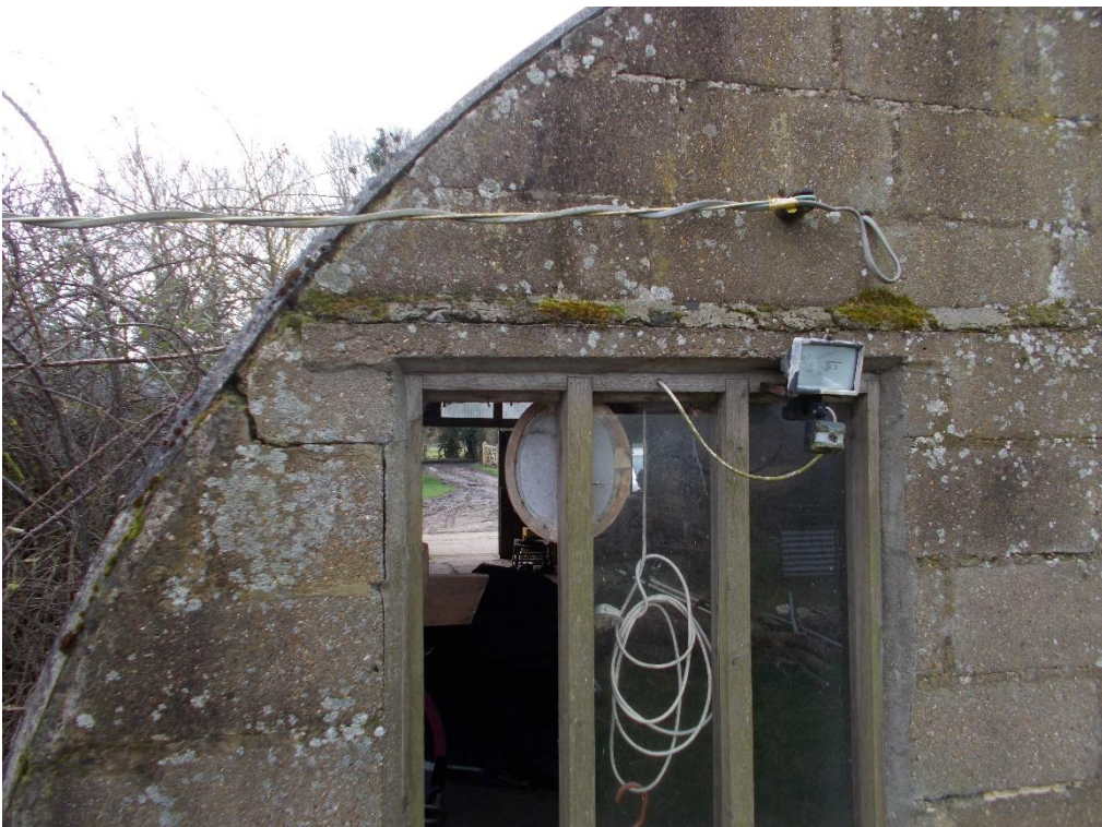
Photograph 6 – Minor lintel movement
