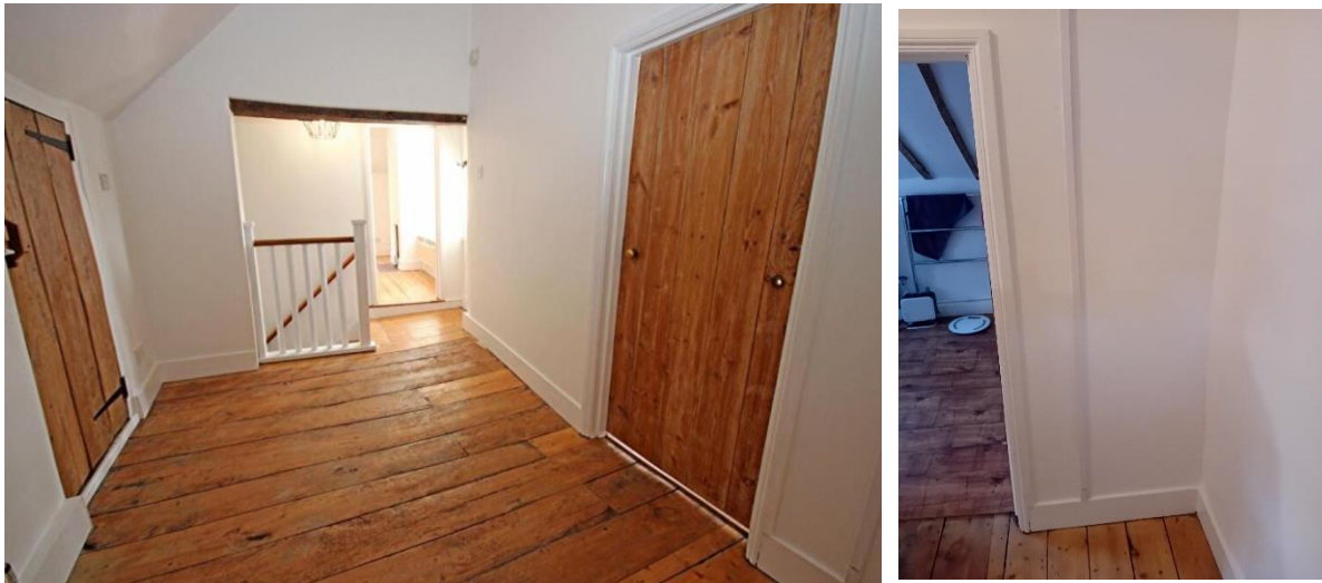
The existing wall between the bathroom and corridor is studwork. This application includes a proposal to reposition part of this wall to enable the enlargement of the existing bathroom. This would improve the usability of the bathroom with minimal impact on the use of the corridor and no detriment to the overall layout or character of the dwelling.
