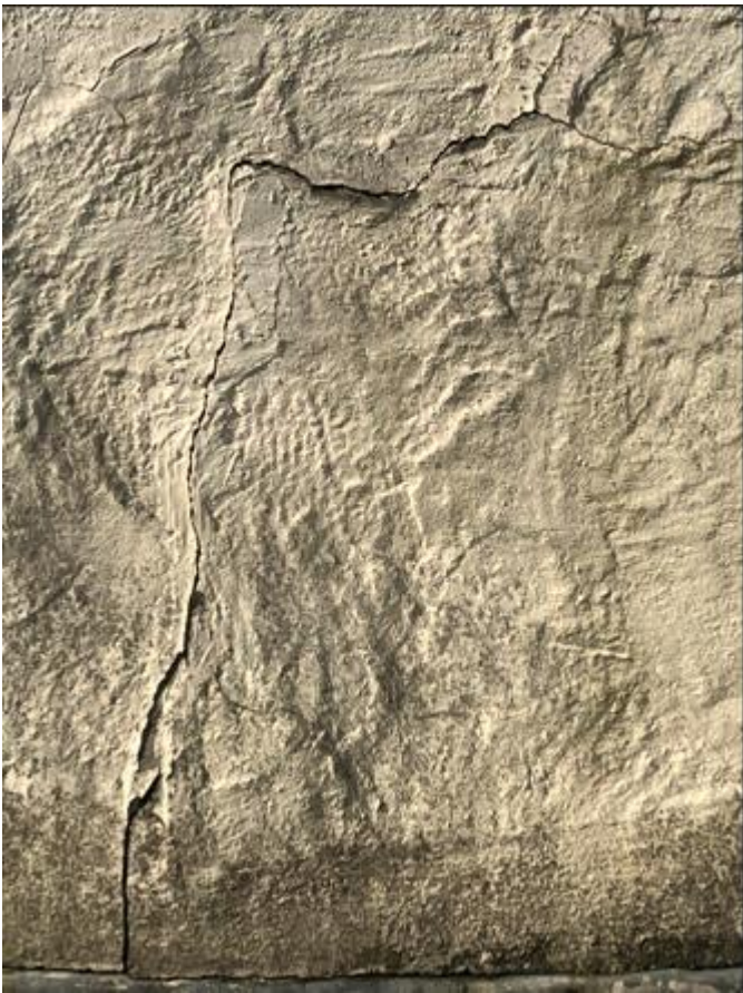
Render has deteriorated beyond repair and is at risk of falling out
