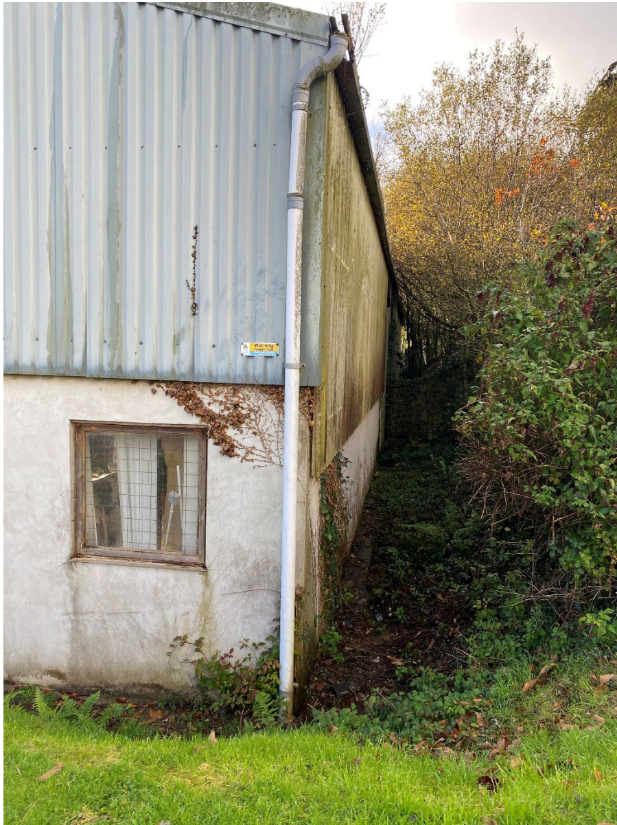
Figure 4: View looking down the side of North elevation of old engineering workshop
