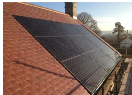
Figure 7 - An example of recessed PV panels
