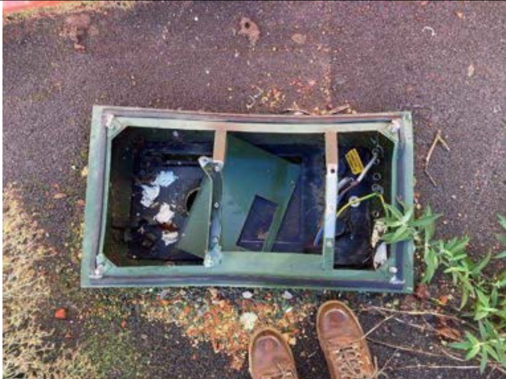
Photograph 5- Electrical box identified within the north-western corner of the site.
