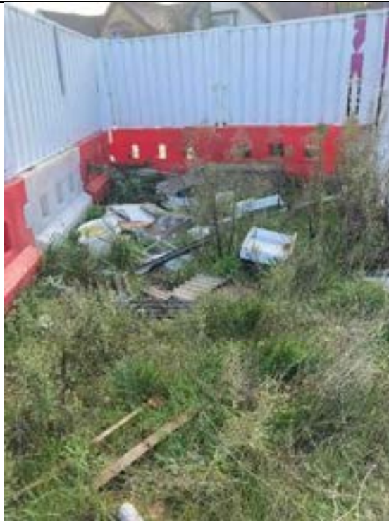
Photograph 6 – South-eastern corner stockpile, containing PACM.
