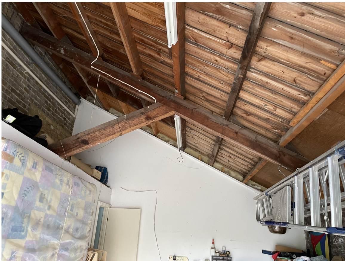
Photograph showing existing timber truss to be left exposed within bedroom and bathroom.
