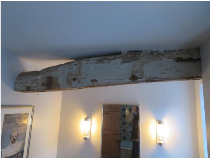
View of beam in bathroom
