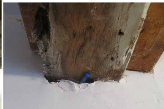
5mm gap under beam where it pass through the partition
