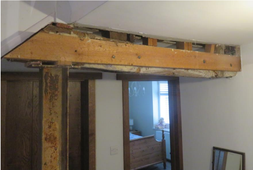
The dropped tie beam cut to accommodate the stairs, is supported on a metal post and repaired using pine flitch plates.
