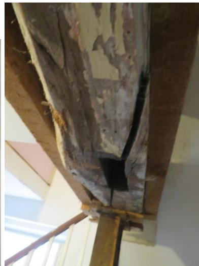
diagonal crack in beam, seen from below
